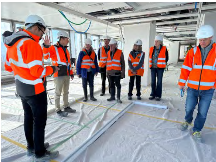
7 th floor: illustrating the floor framework of the office partitioning being fixed in place.
