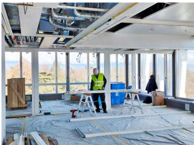
The task of installing the office partitioning has already begun on the 7 th floor.
