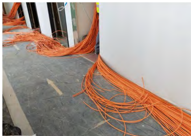
Not a spaghetti factory, just a tiny portion of the 530 Kms of electrical cabling being installed in the Main building.
