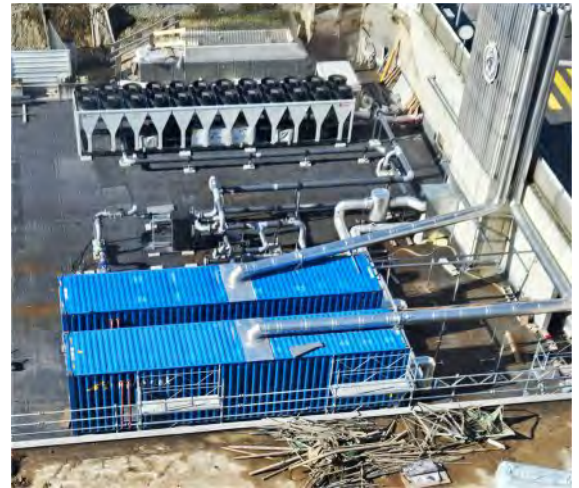
The temporary boilers
