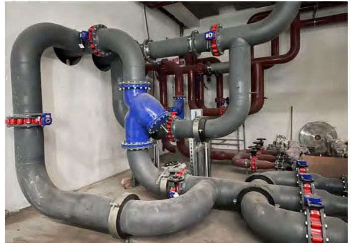
Basement level 3: From the heat exchangers on the other side of the wall, hot and cold water is distributed from here.
