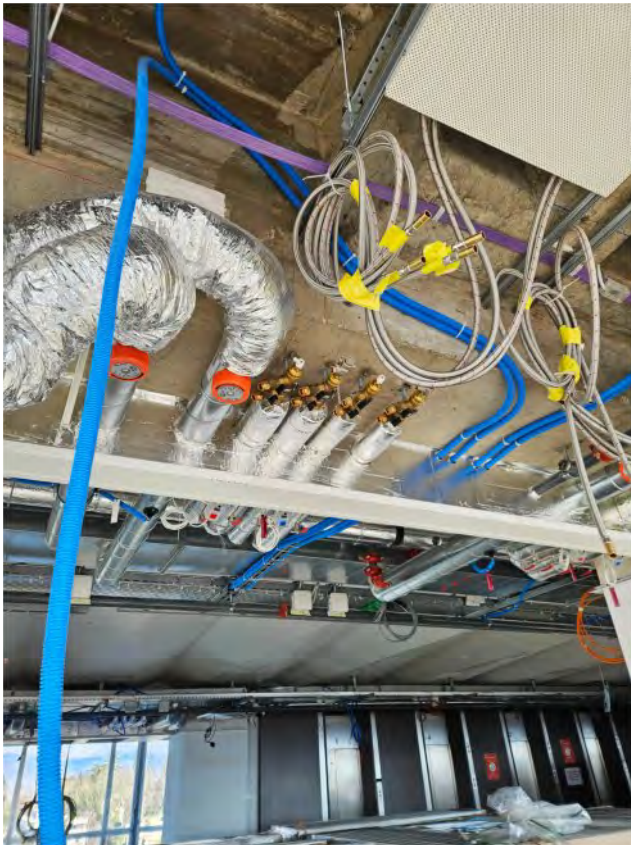
7 th floor: A small idea of the complexity of the restoration that will soon be hidden behind the ceiling panels. The main lifts are in the background.
