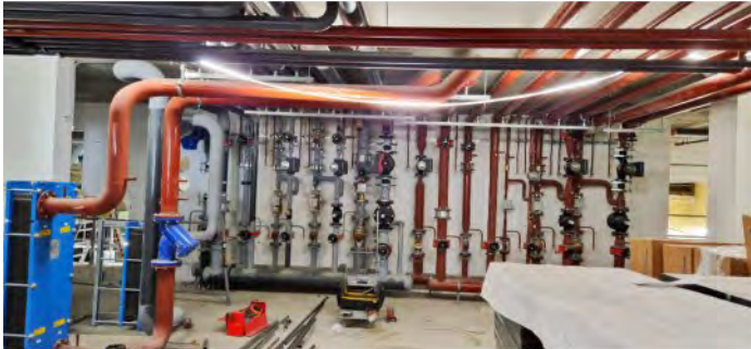
Basement level 3: These smaller bore pipes will then take the hot and cold water to all floors.
