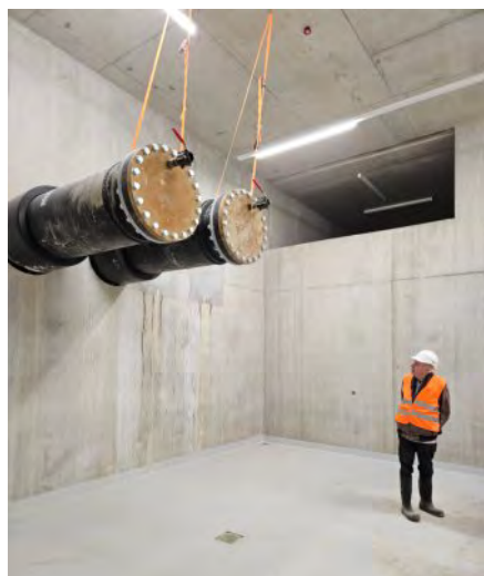
These giant pipes will bring water, pumped from Lake Geneva to WHO, to feed the heat-exchangers.
