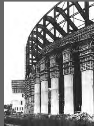
Construction of exterior arches and c deck support beams, 1921, Photos courtesy of University Archives
