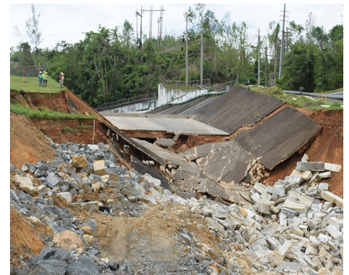
A house (middle right) on the west side of Puerto Rico affected by ocean surge and the damaged spillway of Guajataca Dam (bottom right) Photos courtesy of Daniel Pradel
