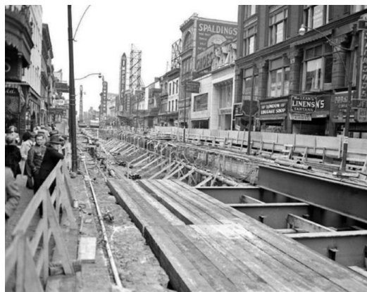
Toronto's Yonge Street subway under construction, using the cut and cover method of construction in the late 1940s (photo source City of Toronto Archives, Series 381, s0381_80015_id6207-3)
