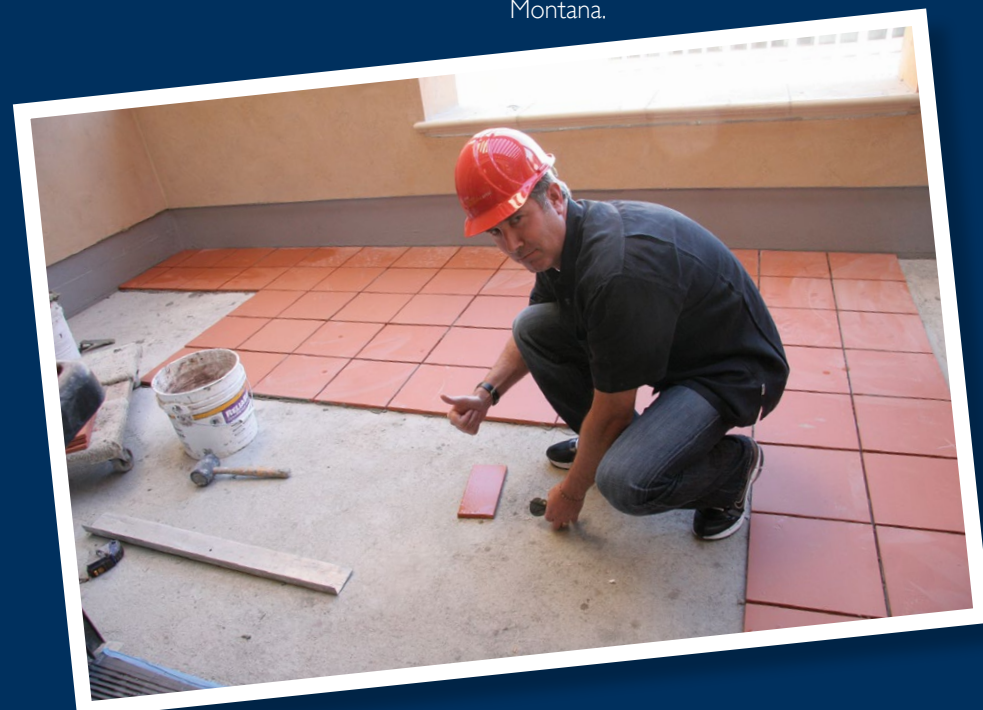
Peter Segal laying tile at the Peter and Linda Segal Balcony at the SCA Complex.
