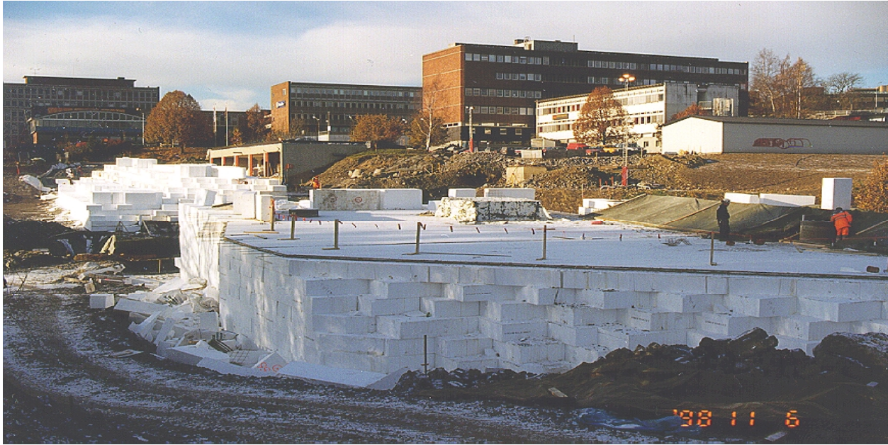
Figure 1. An EPS embankment for a city tramline in Oslo with vertical walls as an alternative to a bridge.
