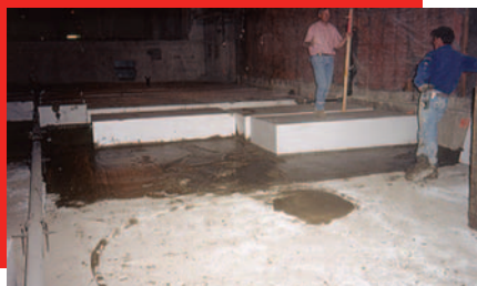
Graphic 5: Filling with blocks of EPS geofoam inside an existing building basement in Chicago, IL [credit: Polyfoam Packers].
