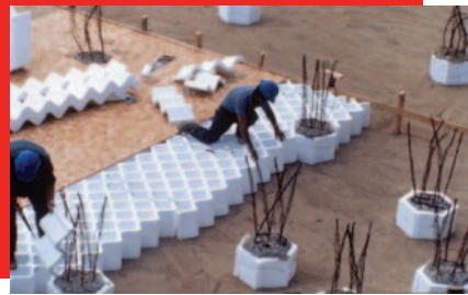
Graphic 6: Placing an EPS-geofoam compressible inclusion (void former) on a building project in Winnipeg, Manitoba, Canada [credit: PFB Corporation/Plasti-Fab Division].
