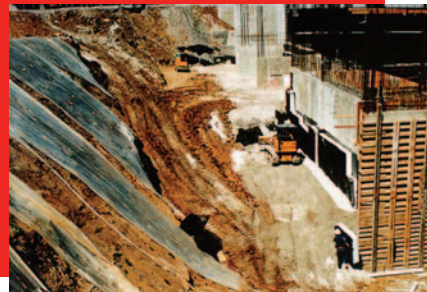
Graphic 7: Use of a multifunctional geofoam compressible inclusion for a deep building basement in Kansas City, MO [credit: GeoTech Systems Corporation].
