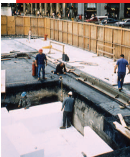
Graphic 3: Below-ground parking structure in Chicago, IL being backfilled with EPS-geofoam blocks on its roof slab [credit: AFM].
