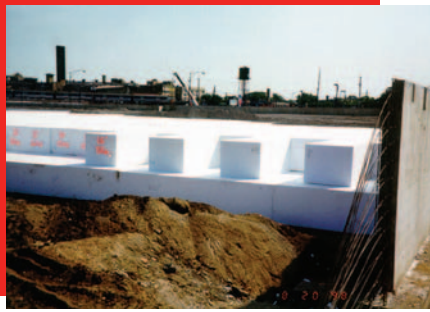
Graphic 4: EPS-geofoam blocks used as both spread-footing foundation support and retaining wall fill for a low-rise commercial building in Chicago, IL [credit: Polyfoam Packers].
