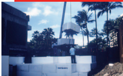
Graphic 2: EPS-geofoam blocks were used in a cramped urban site for a pile-supported hotel in Honolulu, HI [credit: Pacific Allied Products, Ltd.].
