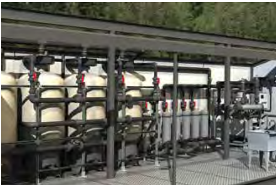
The water treatment process includes dual booster pumps, self-cleaning media filters, cartridge filters, ultraviolet primary disinfection and residual chlorination.
