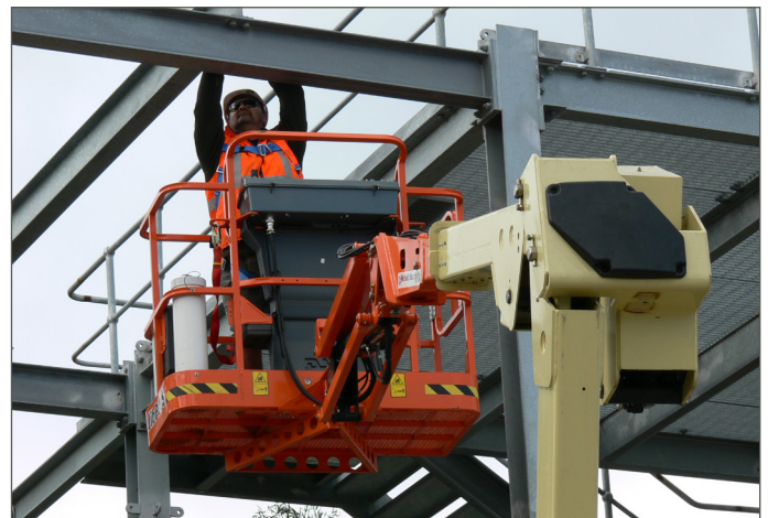
Figure 4. Multiple overhead structures in proximity
