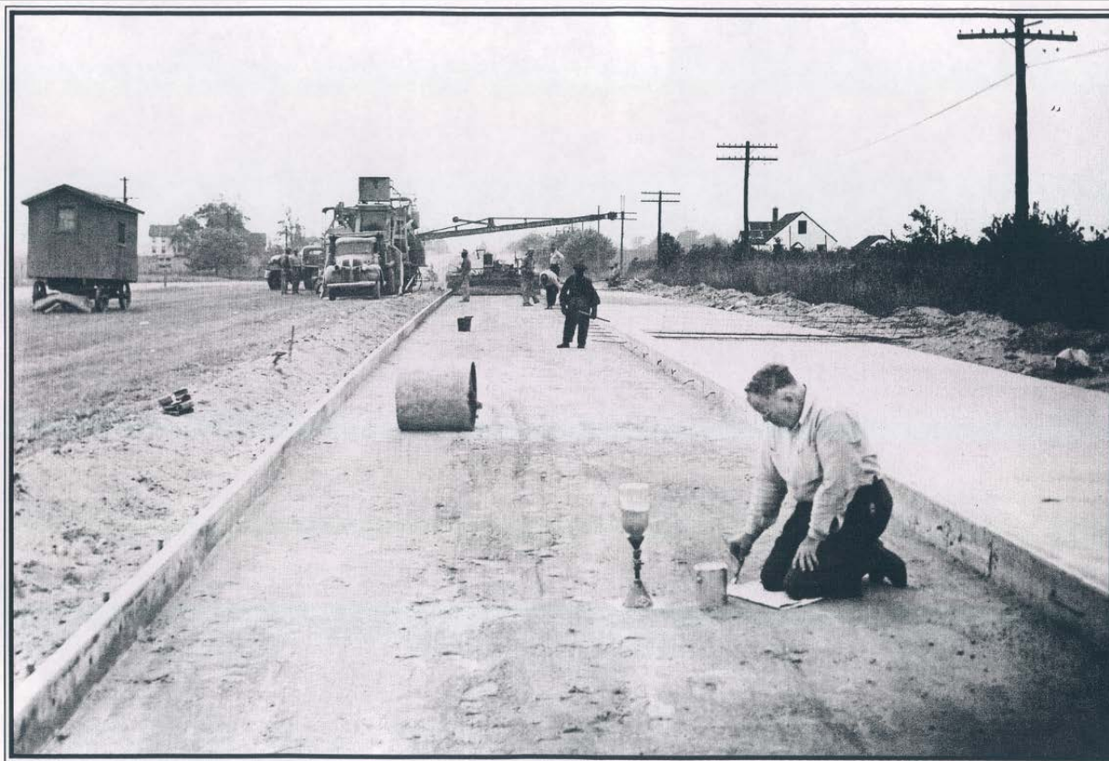
J.W. French conducts a soil density test on the Bear to State Road construction project – 1947
