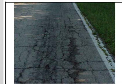
Photo E-18 . Wheel Track Cracking in Local Pavement, High Severity
