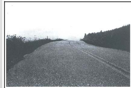
Photo E-14 . Settlement in Local Pavement, Low Severity
