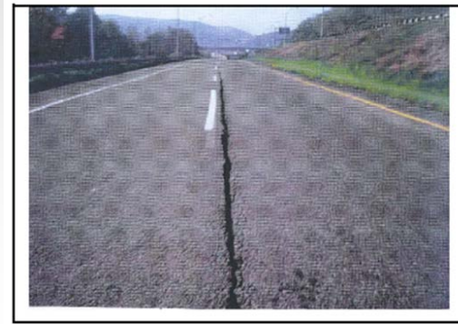
Photo E-20 . Longitudinal Cracking in Local Pavement, High Severity
