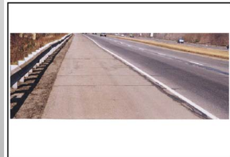
Photo E-15 . Settlement in Local Pavement, Medium Severity
