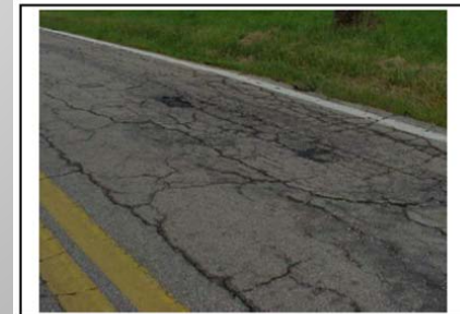
Photo E-19 . Wheel Track Cracking in Local Pavement, High Severity
