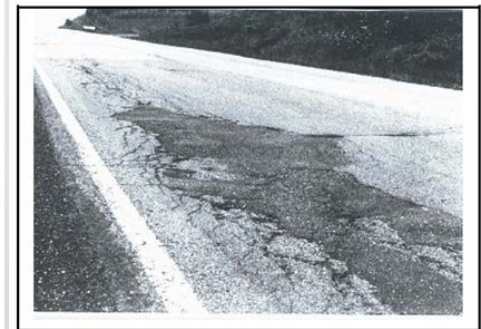
Photo E-5 . Patching in Local Pavement, High Severity
