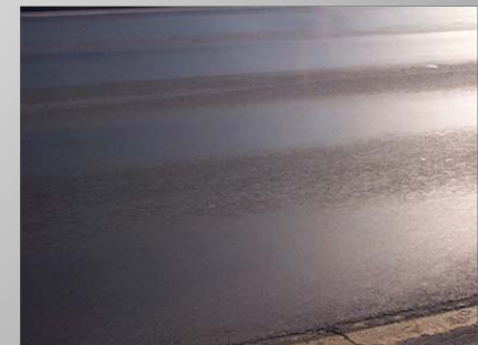
Photo E-4 . Bleeding in Local Pavement, High Severity High Severity shows most aggregates covered with asphalt.
