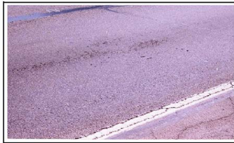
Photo E-1 . Raveling in Local Pavement, Medium Severity
