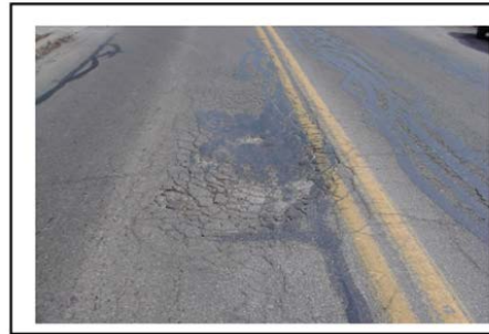
Photo E-13 . Base Failure in Local Pavement, High Severity
