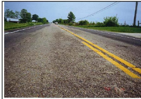
Photo E-2 . Raveling in Local Pavement, High Severity
