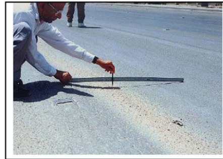
Photo E-10 . Rutting in Local Pavement, High Severity
