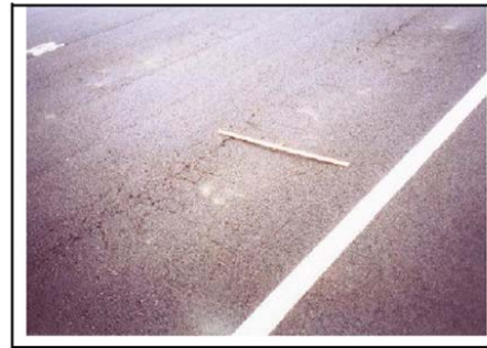
Photo E-9 . Rutting in Local Pavement, Medium Severity
