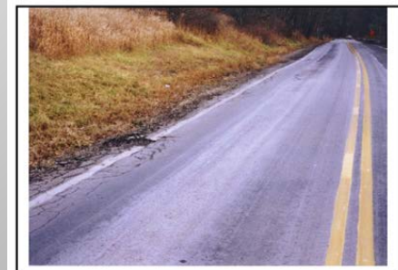
Photo E-22 . Edge Cracking in Local Pavement, High Severity
