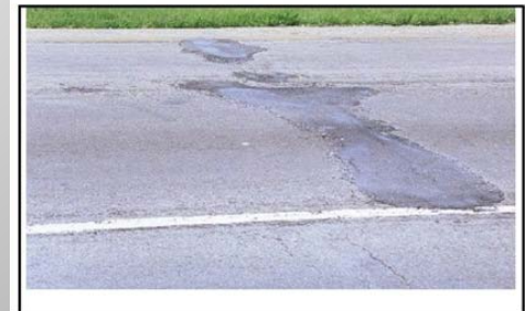
Photo E-6 . Patching in Local Pavement, High Severity
