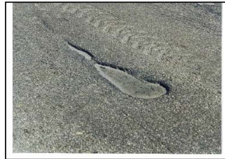
Photo E-8 . Debonding in Local Pavement, Medium Severity
