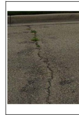
Photo E-17 . Transverse Cracking in Local Pavement, High Severity
