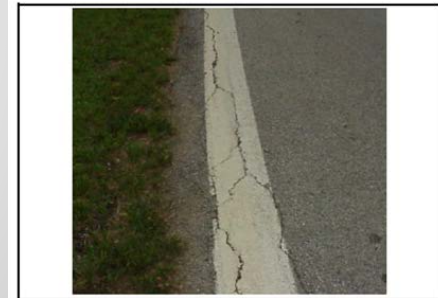
Photo E-21 . Edge Cracking in Local Pavement, Medium Severity
