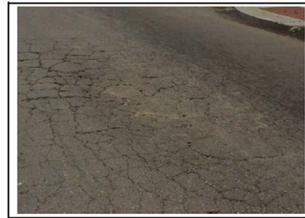
Photo E-12 . Base Failure in Local Pavement, High Severity
