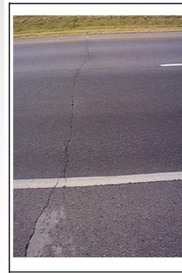
Photo E-16 . Transverse Cracking in Local Pavement, Low Severity
