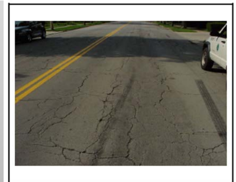
Photo E-11 . Map Cracking in Local Pavement, Medium Severity
