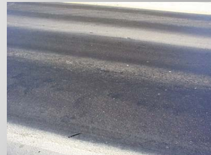
Photo E-3 . Bleeding in Local Pavement, Medium Severity
