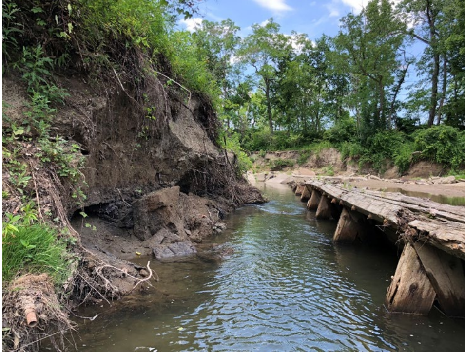
Figure 7. Former City water intake structures contribute to erosion and sedimentation at the mouth of the East Branch. Photo source: Chagrin River Watershed Partners, June 26, 2018.
