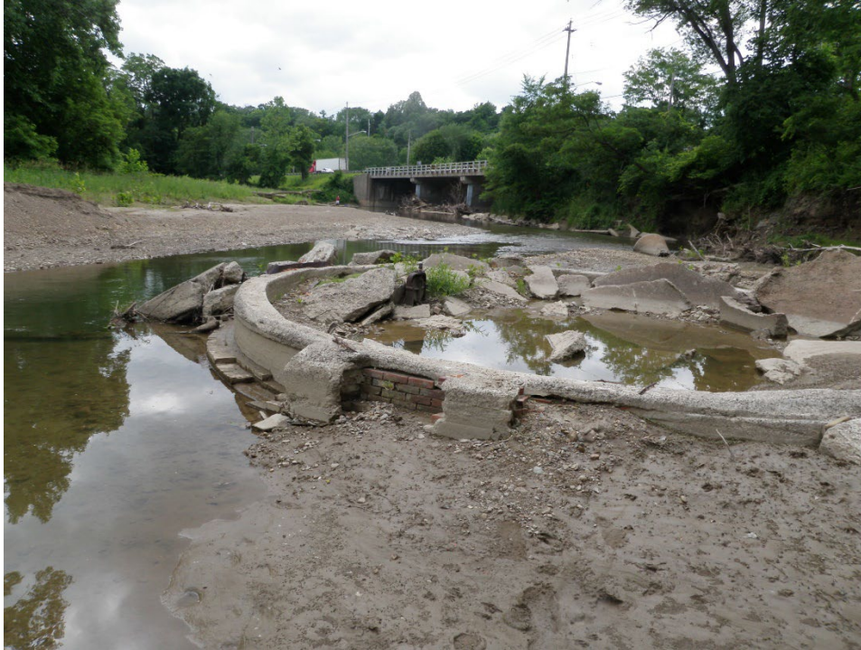
Figure 6. Former City water intake structures contribute to erosion and sedimentation at the mouth of the East Branch. Photo source: Chagrin River Watershed Partners, June 26, 2018.
