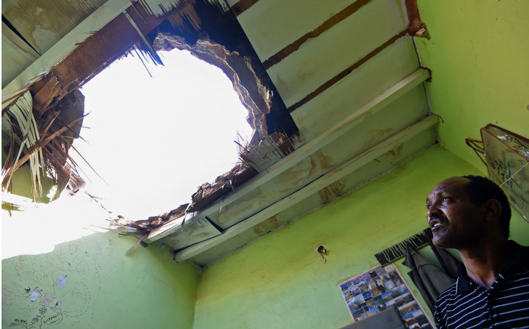
A picture taken March 26, 2018 in Um Al-Hammam district in Riyadh shows a man looking at a hole in a household ceiling caused by falling shrapnel from Yemeni rebel missiles that were intercepted over the Saudi capital.
