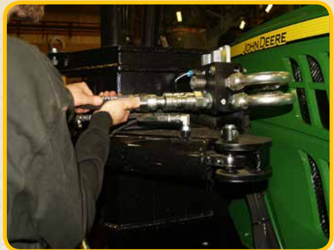
Connect 1" hoses. Wrap hoses in teflon wrap. Wrap is located in the cab of tractor.
