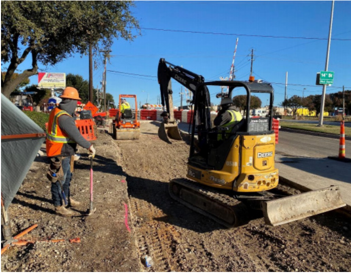
Compacting soil and inserting dowels in prep of paving pour in Plano
