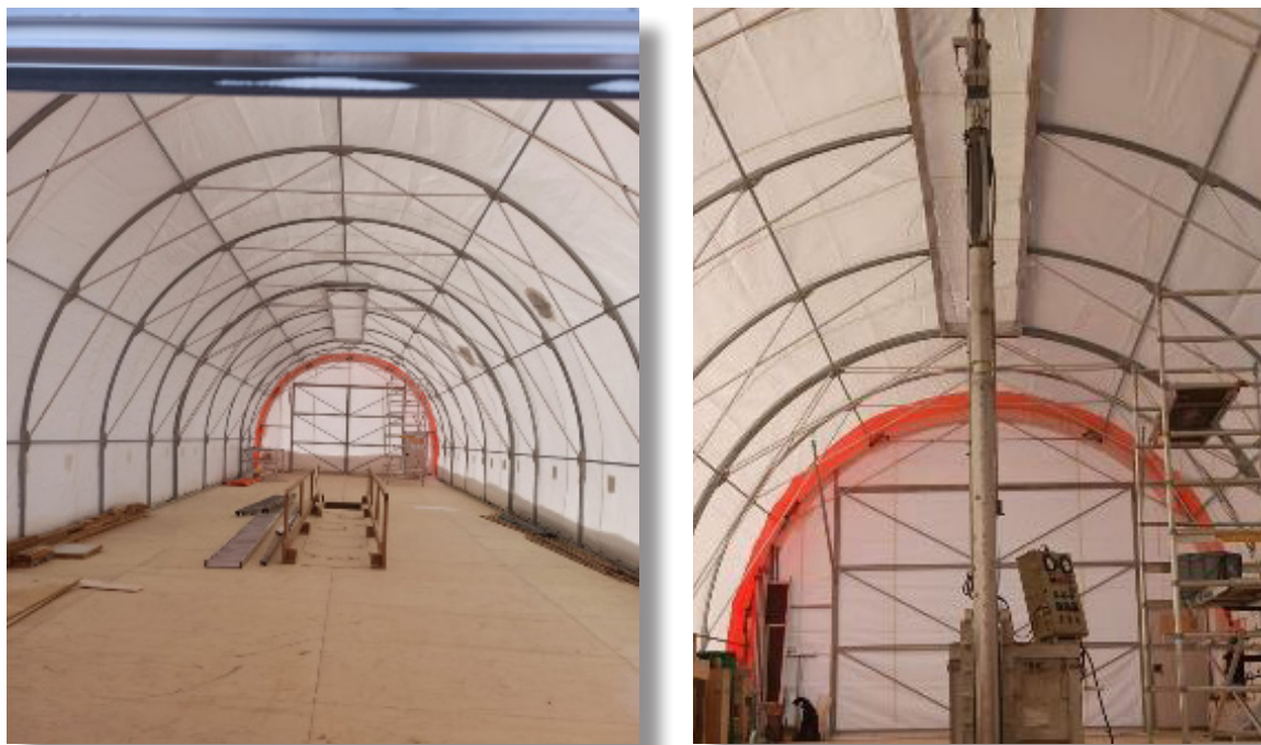
Fig. 7.1.2: The drilling tent at the start of the season (left); installation of the “trapanelle” corer in the tent (right)
