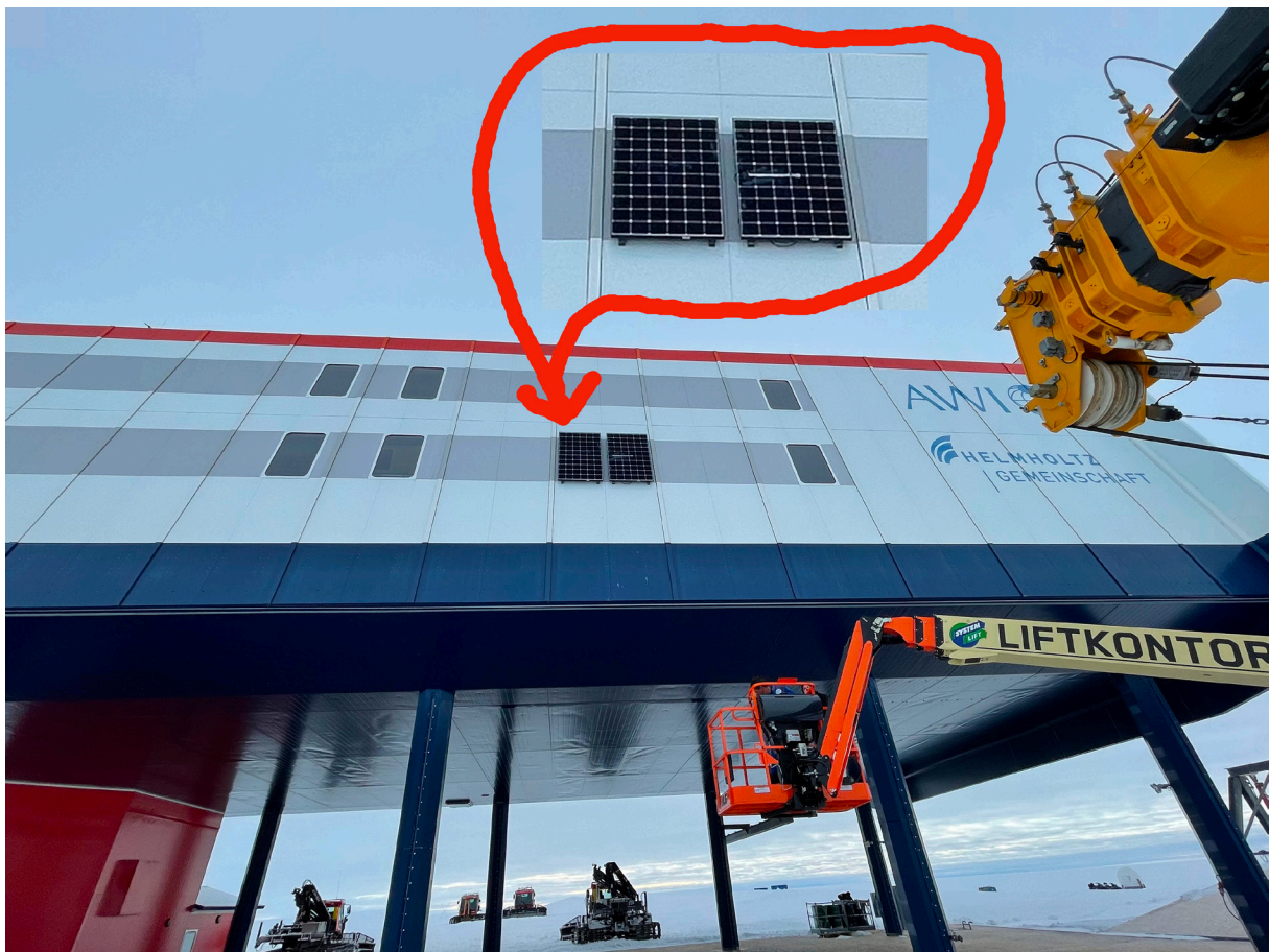
Fig. 3.4.1: Two mounted solar panels on the east side of Neumayer Station III
