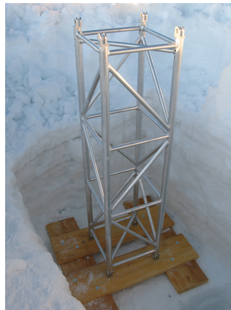
Figure F2. The wooden boards placed at the bottom of the aluminium support tower, at 2 m depth in the firn, during the AWS installation. Photo taken on 30 September 2011.
