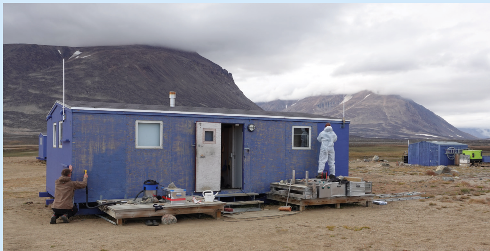
Renovating Zackenberg Research Station in Northeast Greenland involves removing old paint with a 'razor' and a vacuum cleaner to ensure that the old paint is not spread into the environment. Photo: Torben R. Christensen.
