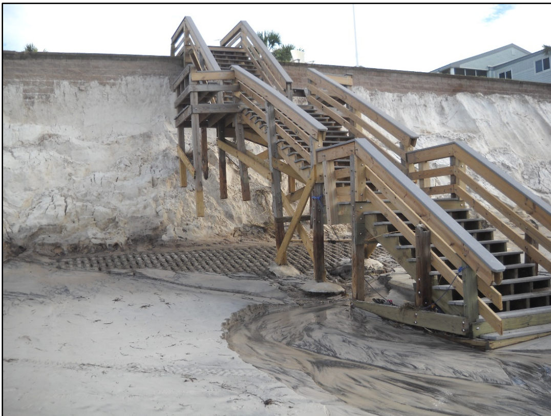
Figure 51. Major dune erosion and exposure of armoring structures, R113.5.
