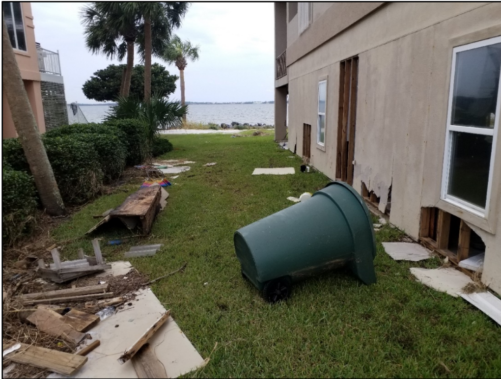
Figure 28. Typical flooding and understructure damage to breakaway walls in Pensacola Beach, R138.
