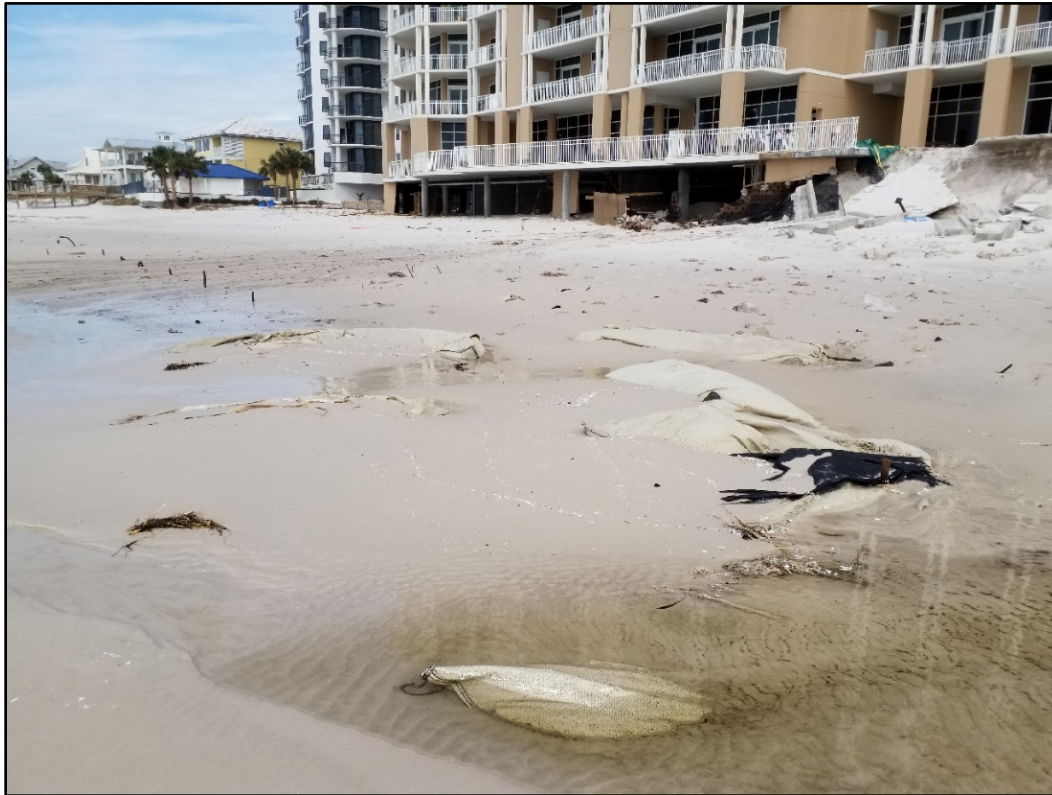
Figure 22. Sand-filled geotextile armoring structure destroyed next to multi-family dwelling with understructure damage, Perdido Key, R32.
