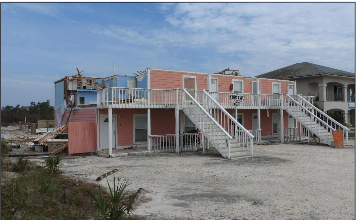
Figure 20. Multi-family dwelling destroyed by wind, Perdido Key, R26.
