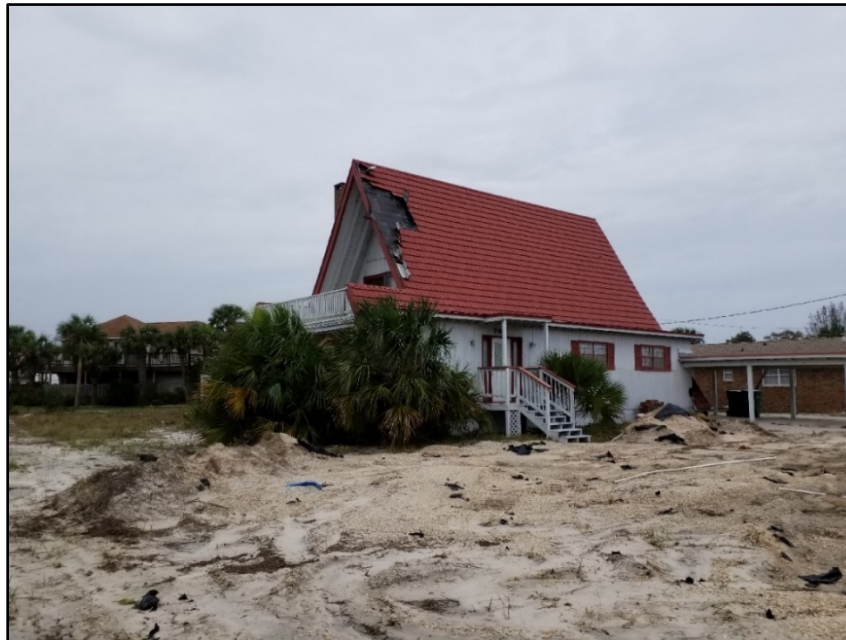
Figure 43. Typical roof damage in Okaloosa Island, R4.
