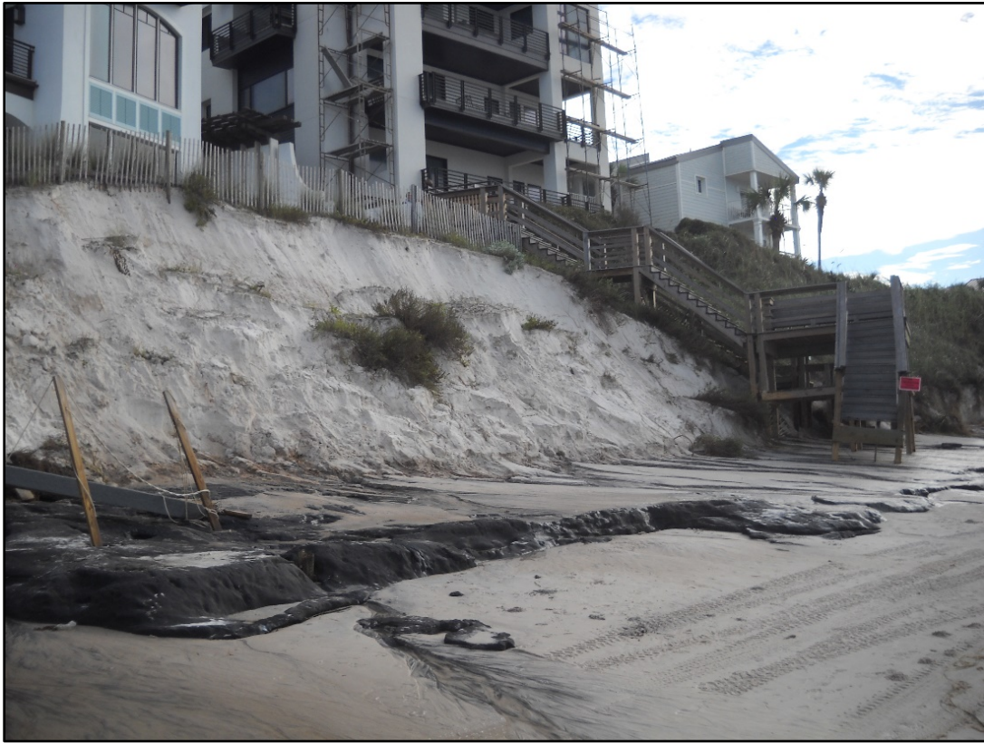
Figure 50. Major dune erosion exposing peat layer in Seacrest Beach, R113.
