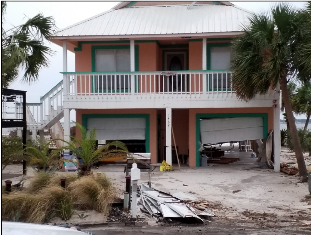
Figure 35. Understructure damage, Navarre Beach, R203.5.
