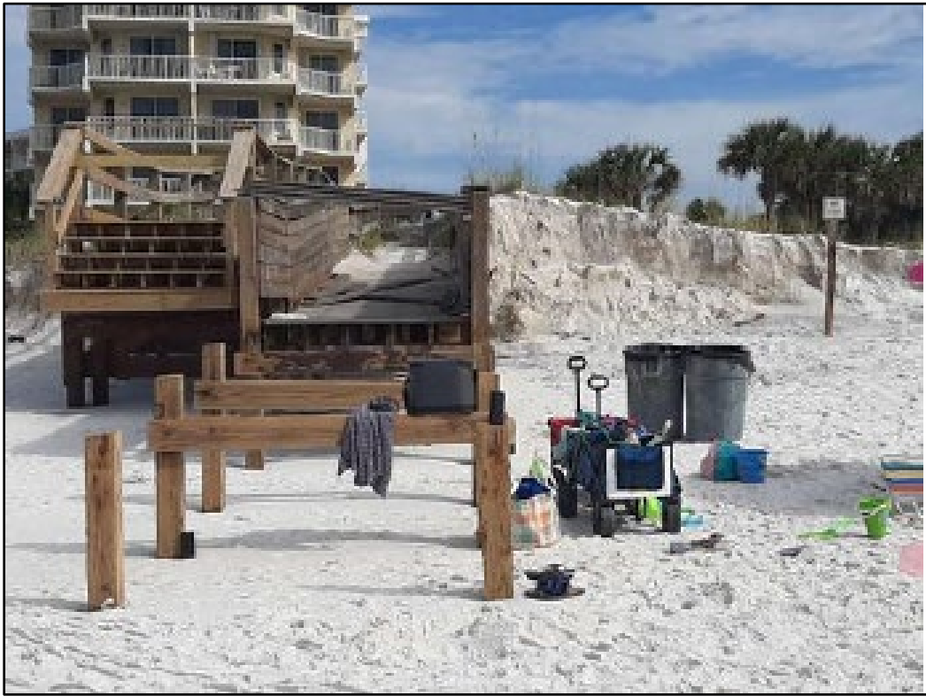
Figure 39. Moderate beach and dune erosion in Okaloosa Island, R114.5.
