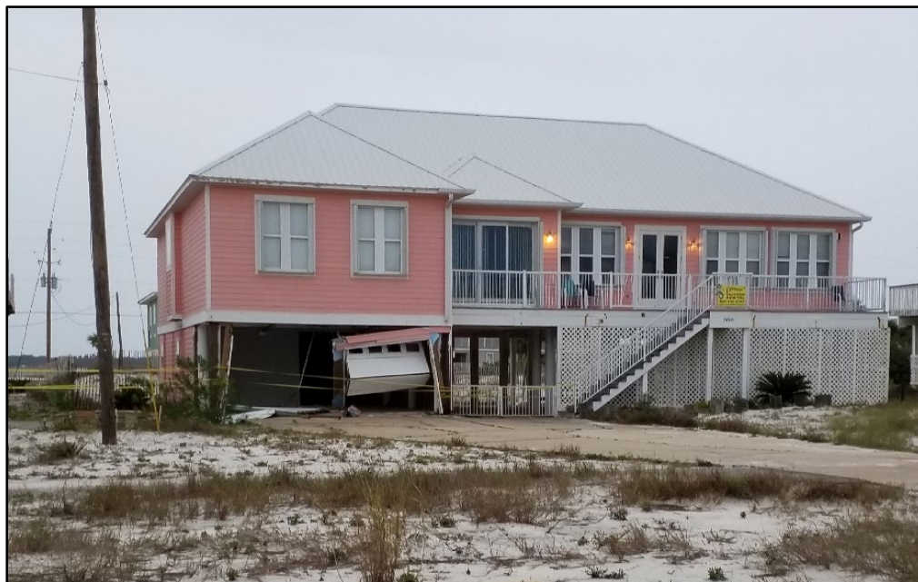
Figure 34. Typical understructure damage due to the storm surge, Navarre Beach, R195.
