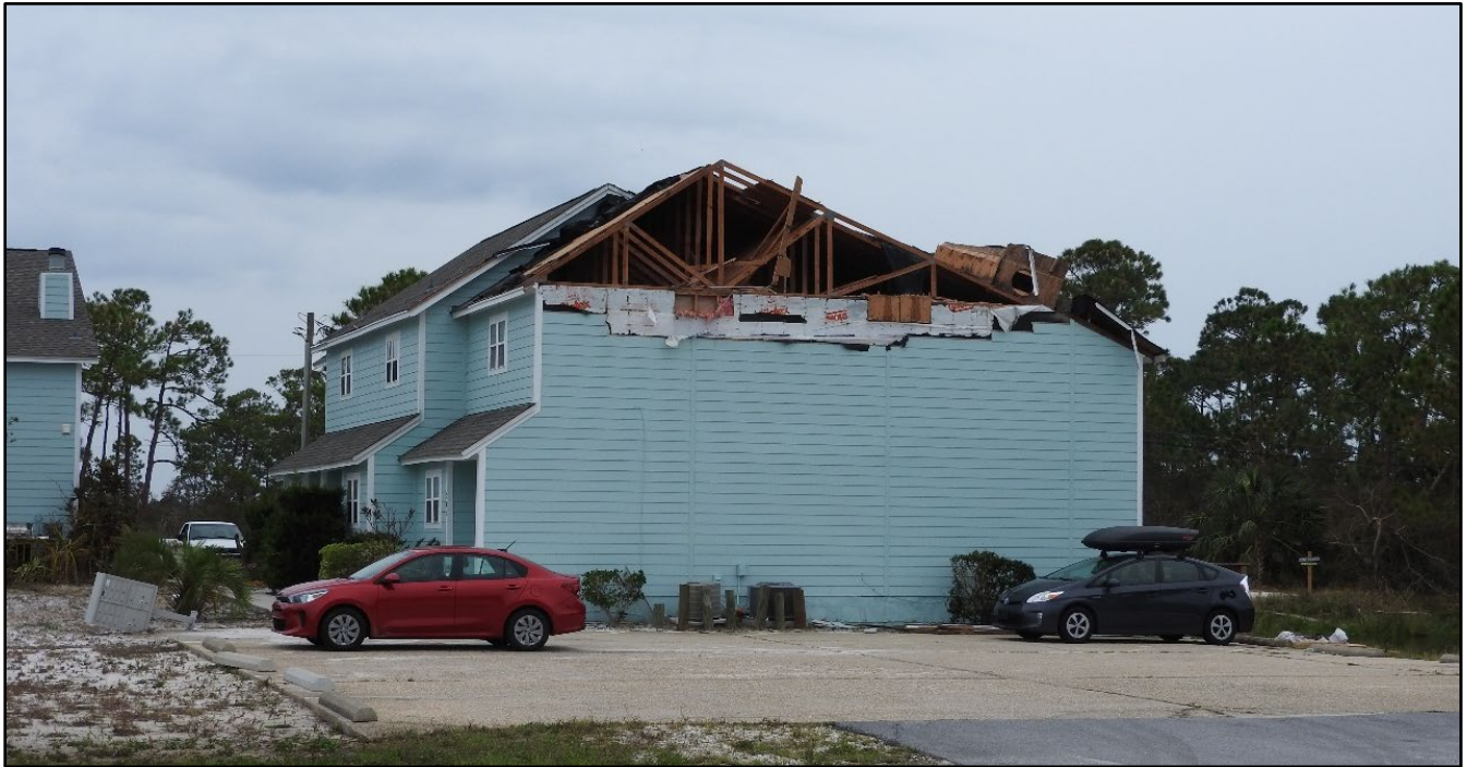
Figure 24. Major roof damage to multi-family building, Perdido Key.
