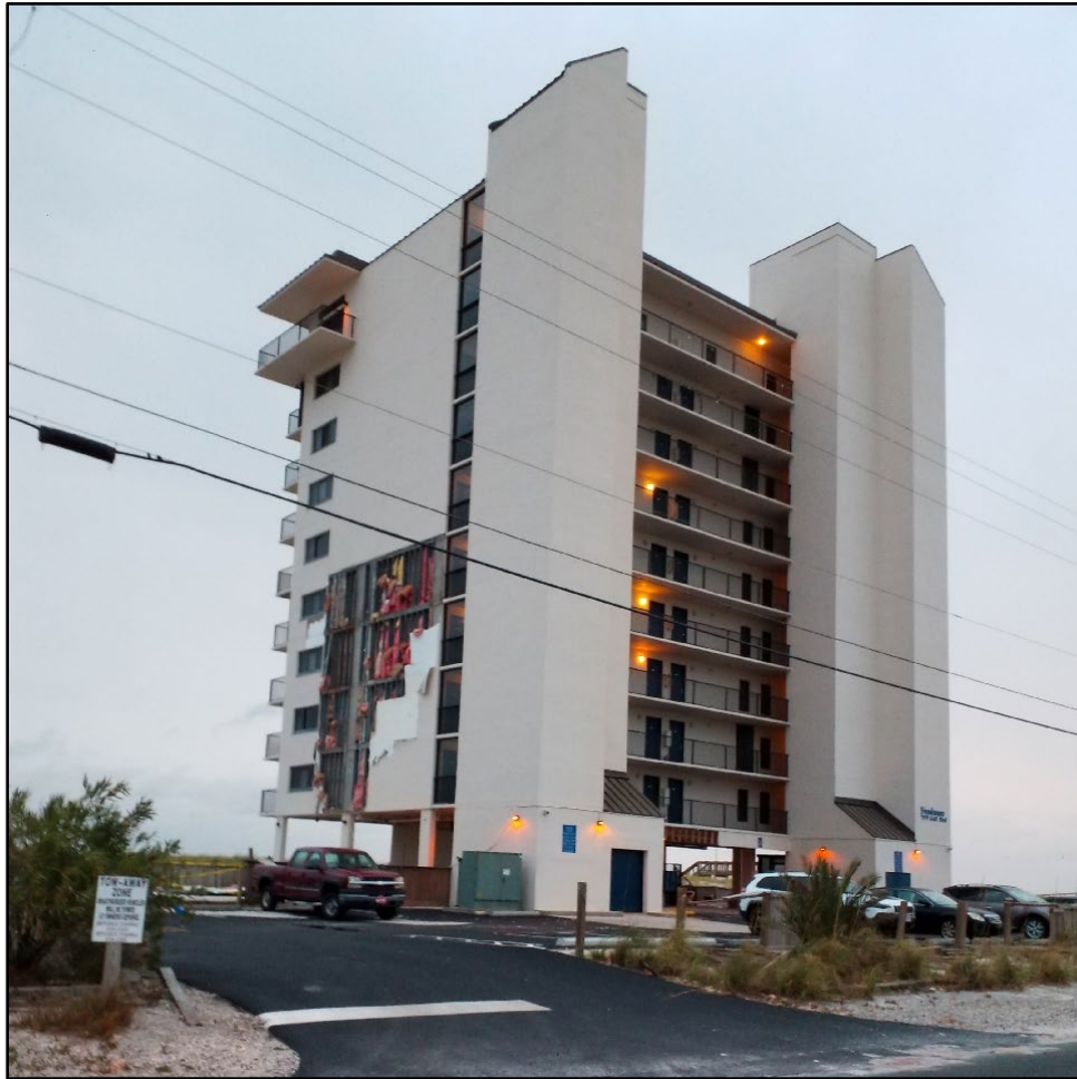
Figure 33. Major siding damage to a multi-family building, Navarre Beach, R201.5.
