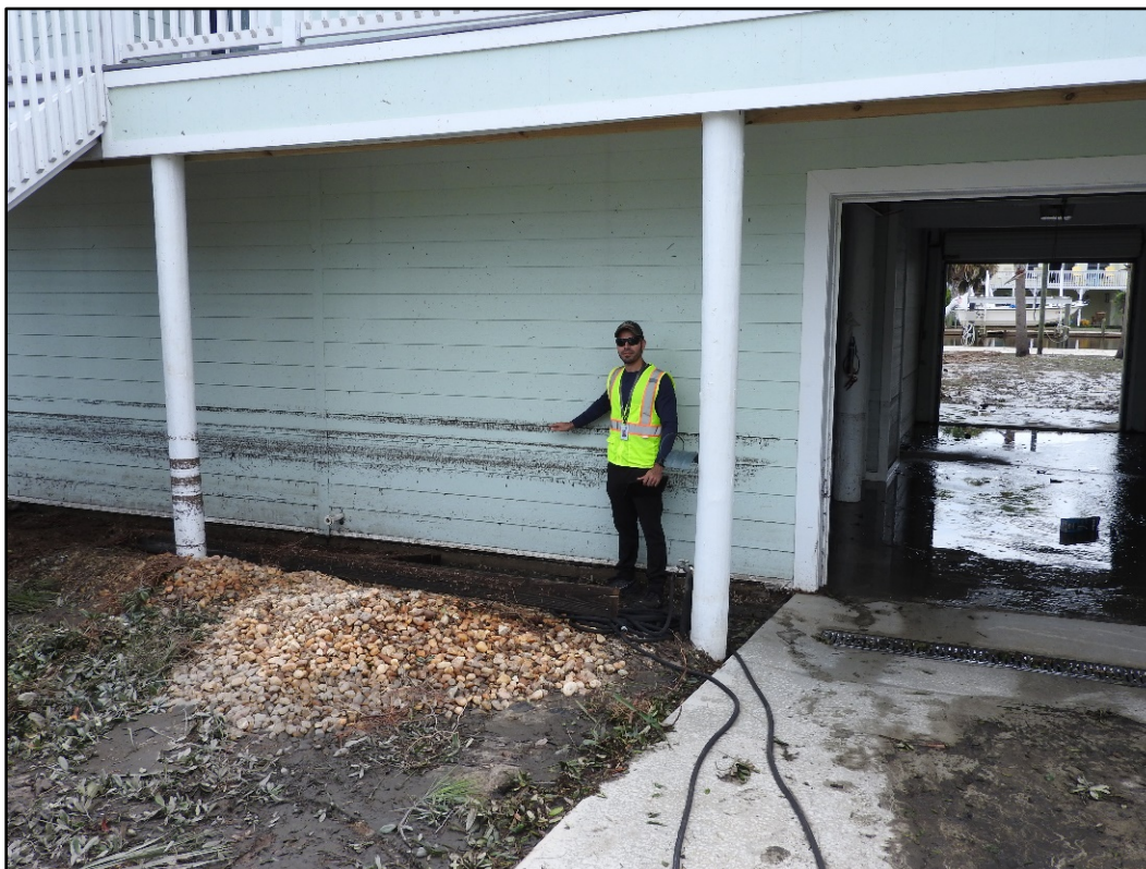
Figure 23. Typical flooding at ground level, Perdido Key.
