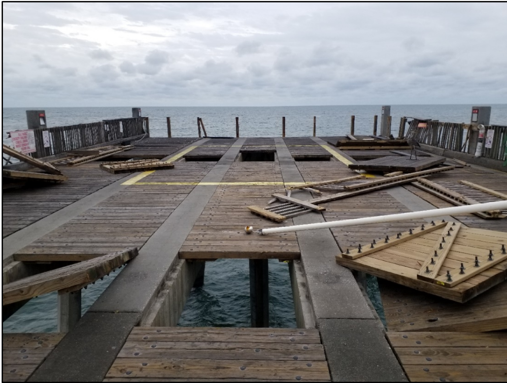
Figure 26. Pensacola Beach Fishing Pier with breakaway deck sections and handrails displaced, but no major structural damage, R120.5.
