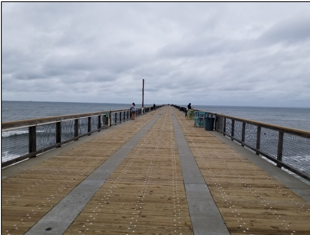
Figure 36. No damage to the Navarre Fishing Pier, the longest pier on the Gulf of Mexico, R209.5.
