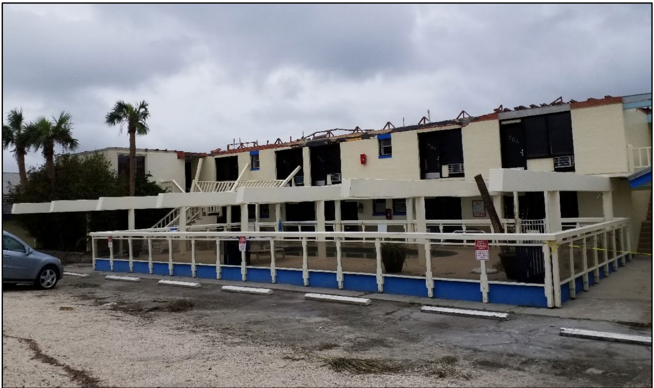
Figure 25. Major roof damage on the Pensacola Inn, Pensacola Beach, R123.
