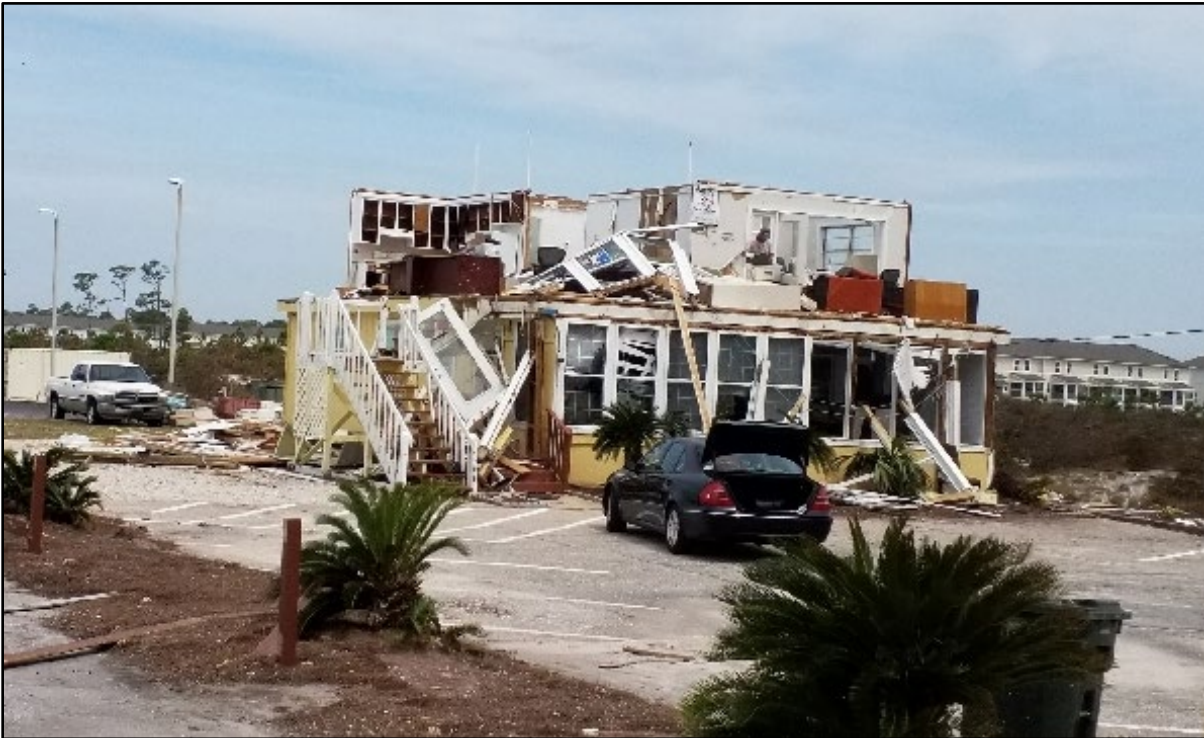
Figure 19. Commercial building destroyed by wind, Perdido Key, R24.
