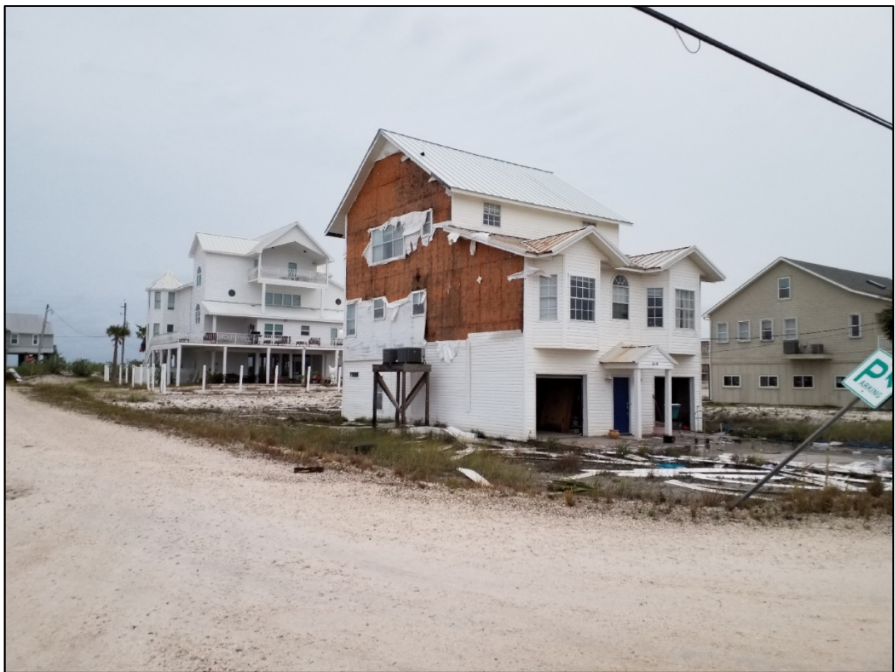
Figure 32. Major siding damage to a single family dwelling, Navarre Beach, R203.
