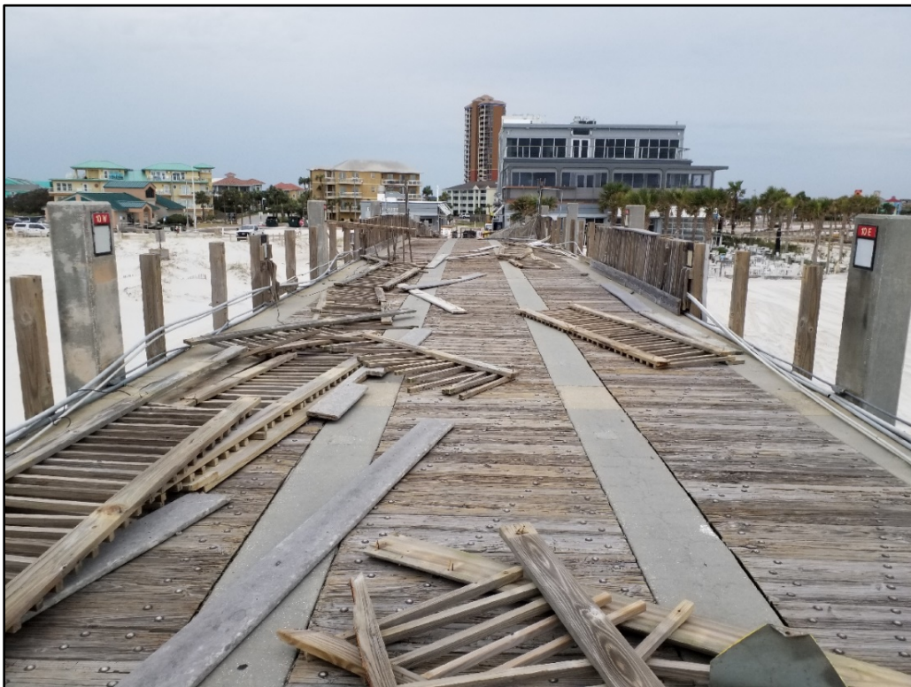
Figure 27. Pensacola Beach Fishing Pier with breakaway handrails displaced, but no major structural damage, R120.5.
