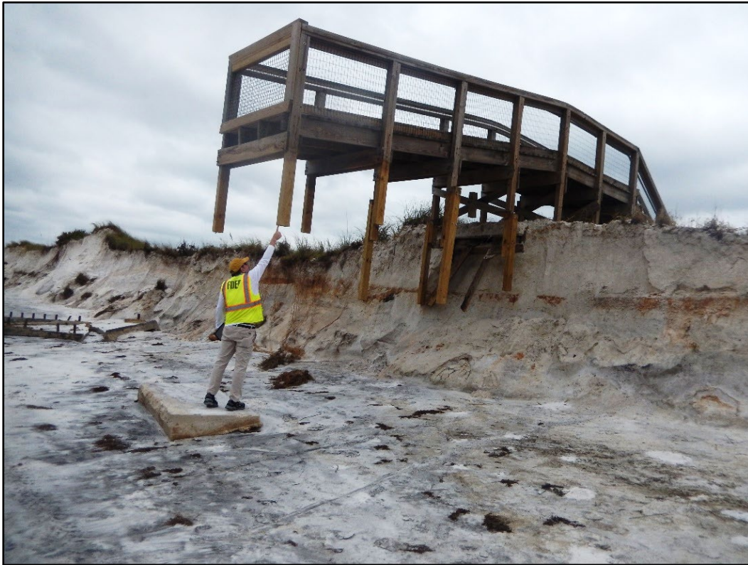
Figure 59. Major dune erosion with park infrastructure damage (R96) following Hurricane Sally.
