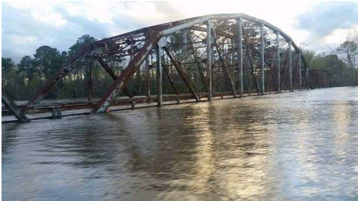
Burr's Ferry Bridge SH 63 over Sabine River – photo by Texas Department of Transportation
