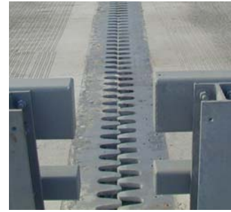
PHOTO 11: Bascule Leaf Transverse Joint
