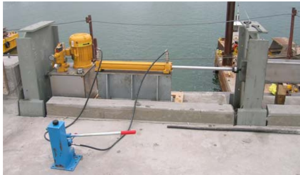
PHOTO 27: Span Lock Hydraulic Cylinder Actuator and Power Unit
