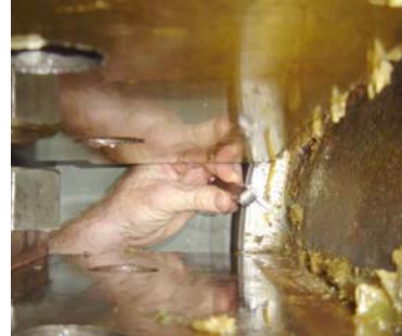
PHOTO 14: Trunnion Bearing Feeler Gauge Measurements
