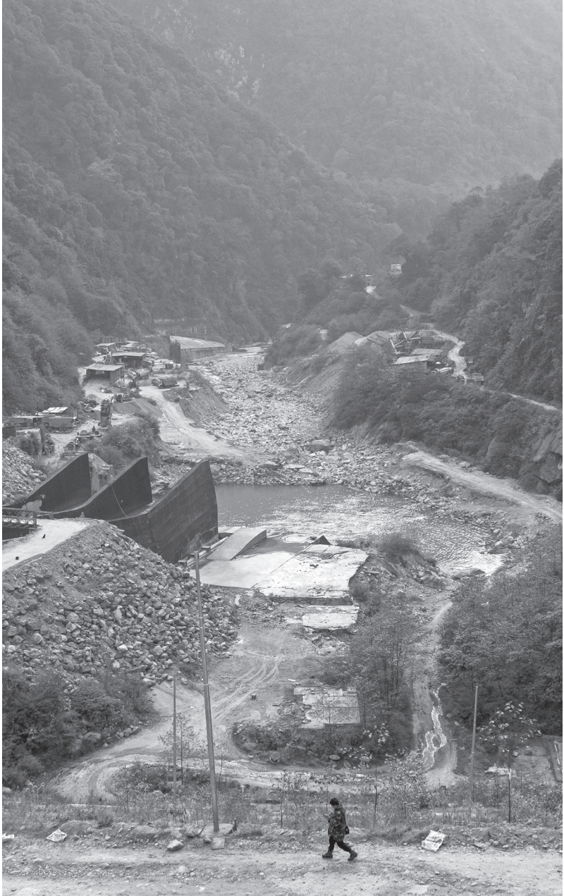
Teesta, as it struggles out of the Stage-III HEP at Chungthang in North Sikkim
