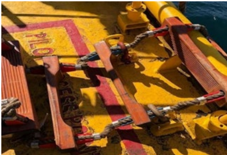
Photo 4: Unsafe pilot ladder securing arrangements (Reproduced with permission from Fremantle Ports). Photo credit: AMSA
