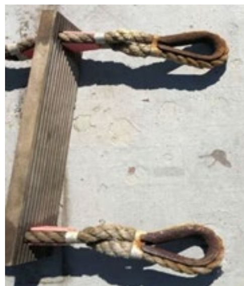
Photo 9: Example of corroded end point thimbles (Reproduced with permission from Fremantle Ports). Photo credit: AMSA
