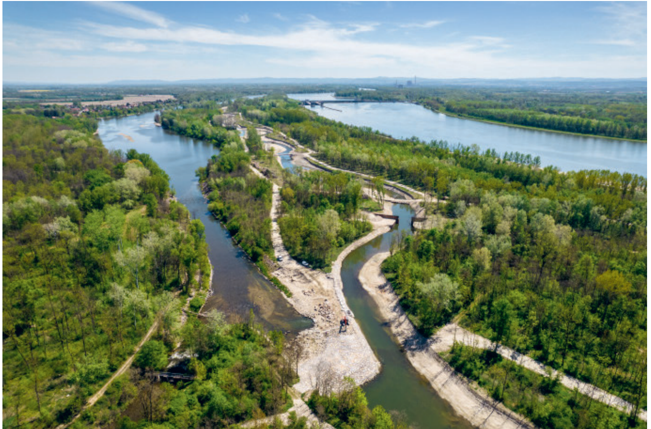
Fish migration facility at the power plant Altenwörth during the construction phase
