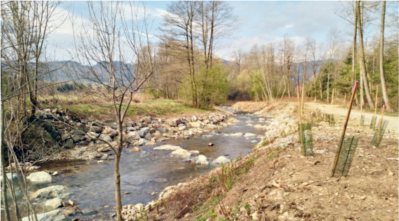
Restored river gradient in the area of the former transverse structure in Kerschbaum
