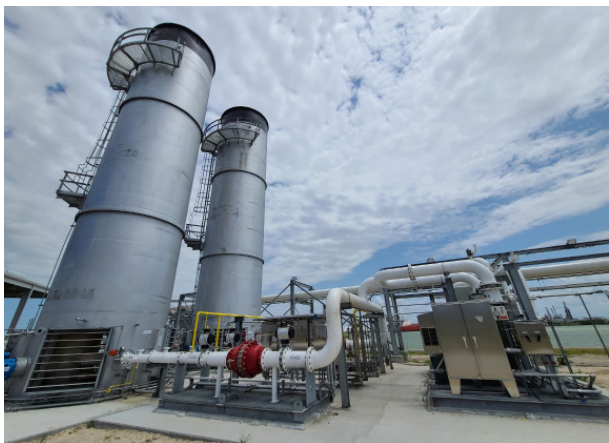
Figure 1. Typical marine vapour combustion system in operation on the US Gulf Coast.
