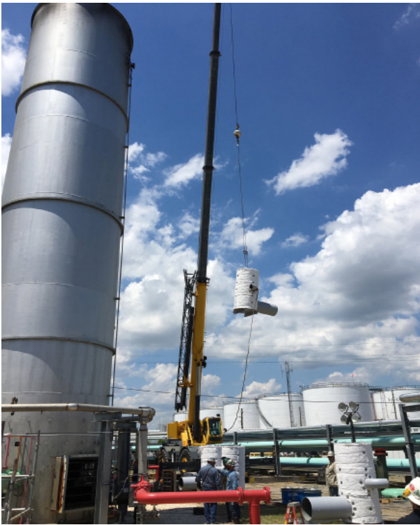
Figure 4. Existing vapour combustion unit undergoing retrofit for improved capacity and performance.
