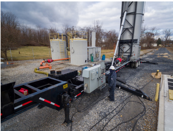
Figure 5. Zeeco portable vapour combustion unit in use during maintenance of a vapour recovery unit.
