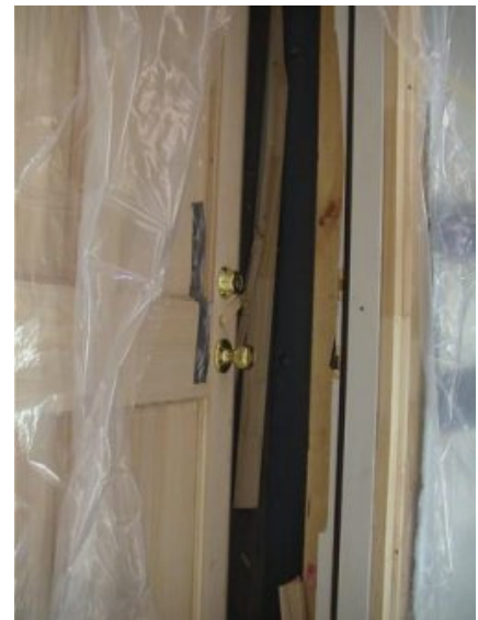
This un-reinforced door frame gave way at the strike plate when the door was subjected to wind pressures. The vinyl sheeting was used to help apply the pressure.
