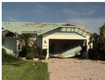
Garage door blown in on top of car. Note the loss of roof sheathing over the garage.
