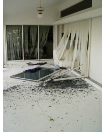
The failure of French doors at the front of this house resulted in the sliding glass doors being blown out of their tracks. Note one of the tempered glass panels did not break.
