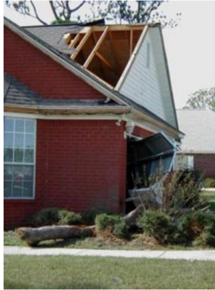
The failure of this garage door probably contributed to the loss of roof sheathing.
