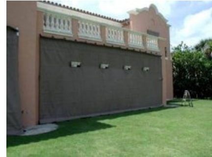
A screen product protecting an entire porch area keeps water away from doors and prevents a sudden in rush of wind.
