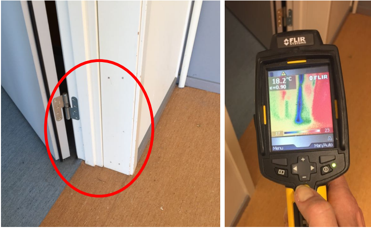
Figure 5.7: To the left is a photograph and to the right is a thermography of air leakage location L4. The air is leaking through cracks in the connection of the door frame to the inner wall and floor.
