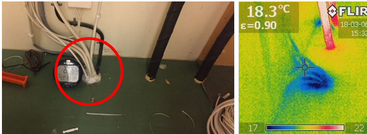
Figure 5.6: To the left is a photograph and to the right is a thermography of air leakage location L1. The air is leaking through a penetration through the floor construction in which electrical wires are installed.
