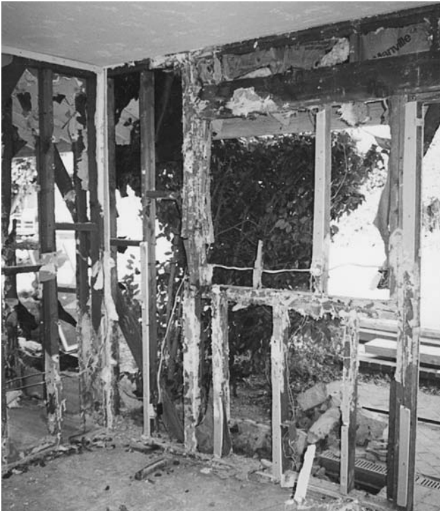
Fig. 14.2. Extensive dry rot of timber frame of home in California caused by Meruliporia incrassata . Damage occurred during construction. Photograph courtesy of Luis De La Cruz (De La Cruz Wood Preservation Services, Van Nuys, CA).
