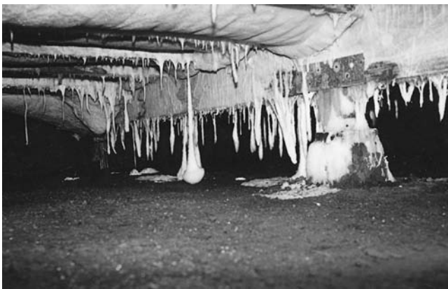
Fig. 14.6. Wood decay in recently constructed home by unidentified wet rot fungus. Photograph courtesy of Luis De La Cruz (De La Cruz Wood Preservation Services, Van Nuys, CA).
