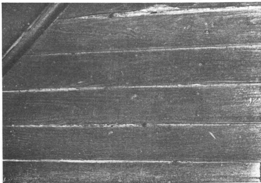
F-512969 Figure 6.—During dry weather, shrinkage cracks in floors often outline extent of attack by Poria incrassata .
