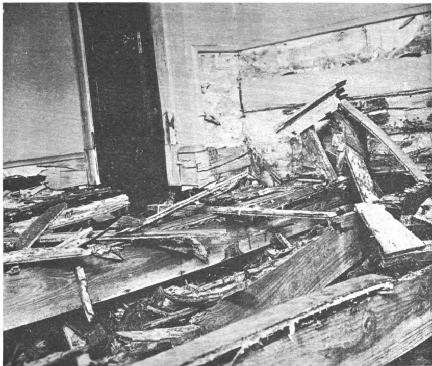
M-19037 F Figure 5.—Framing, flooring, joists, and trim of house decayed by Poria incrassata .
