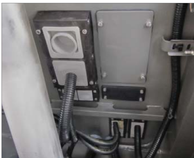
KEL-JUMBO 2 - Page 34 / KEL 24|x - Page 18 Routing of conduits and large cables between vehicle body and chassis
