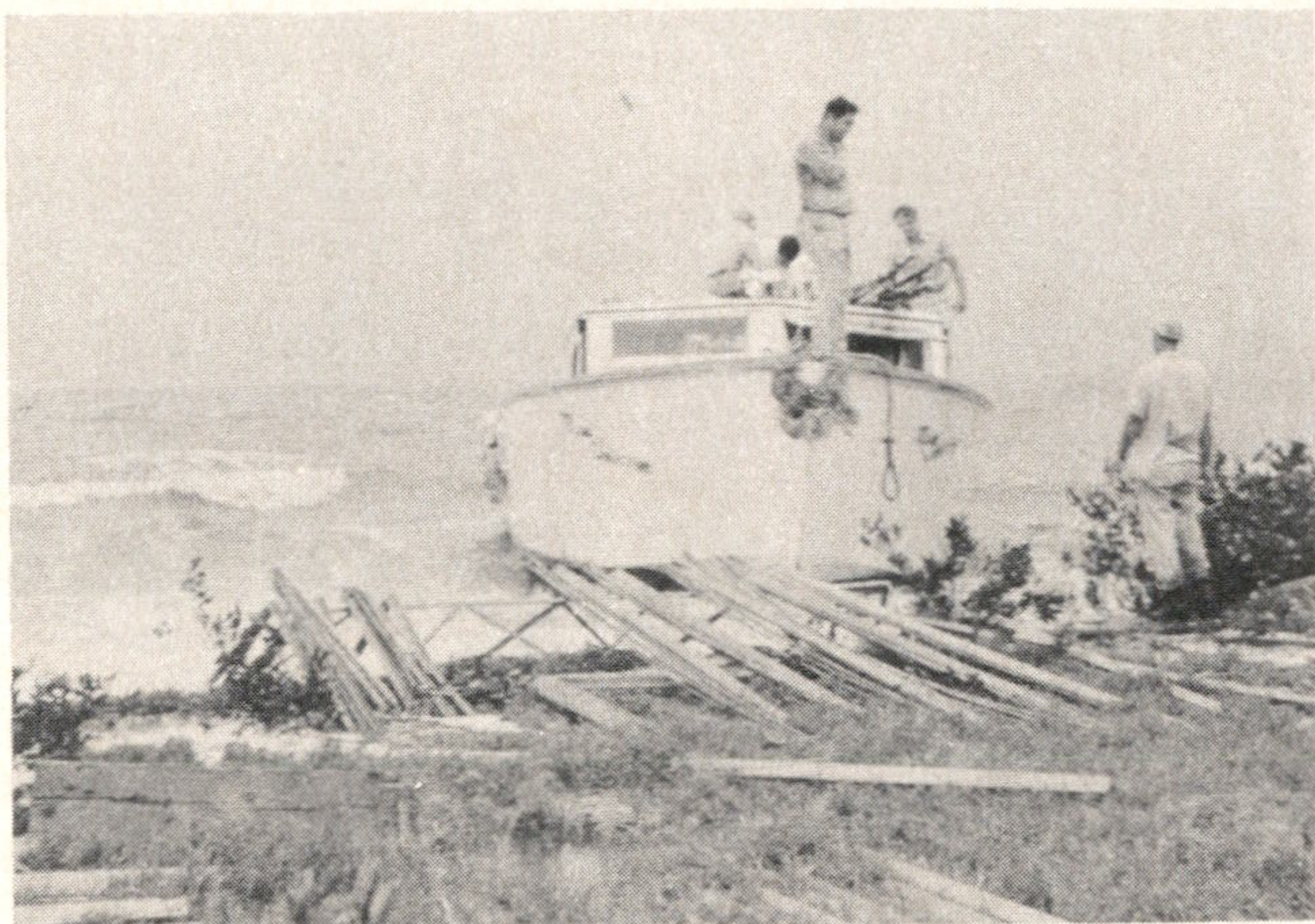
Unloading operations of tower members. Note roughness of water and boat being completely aground.
