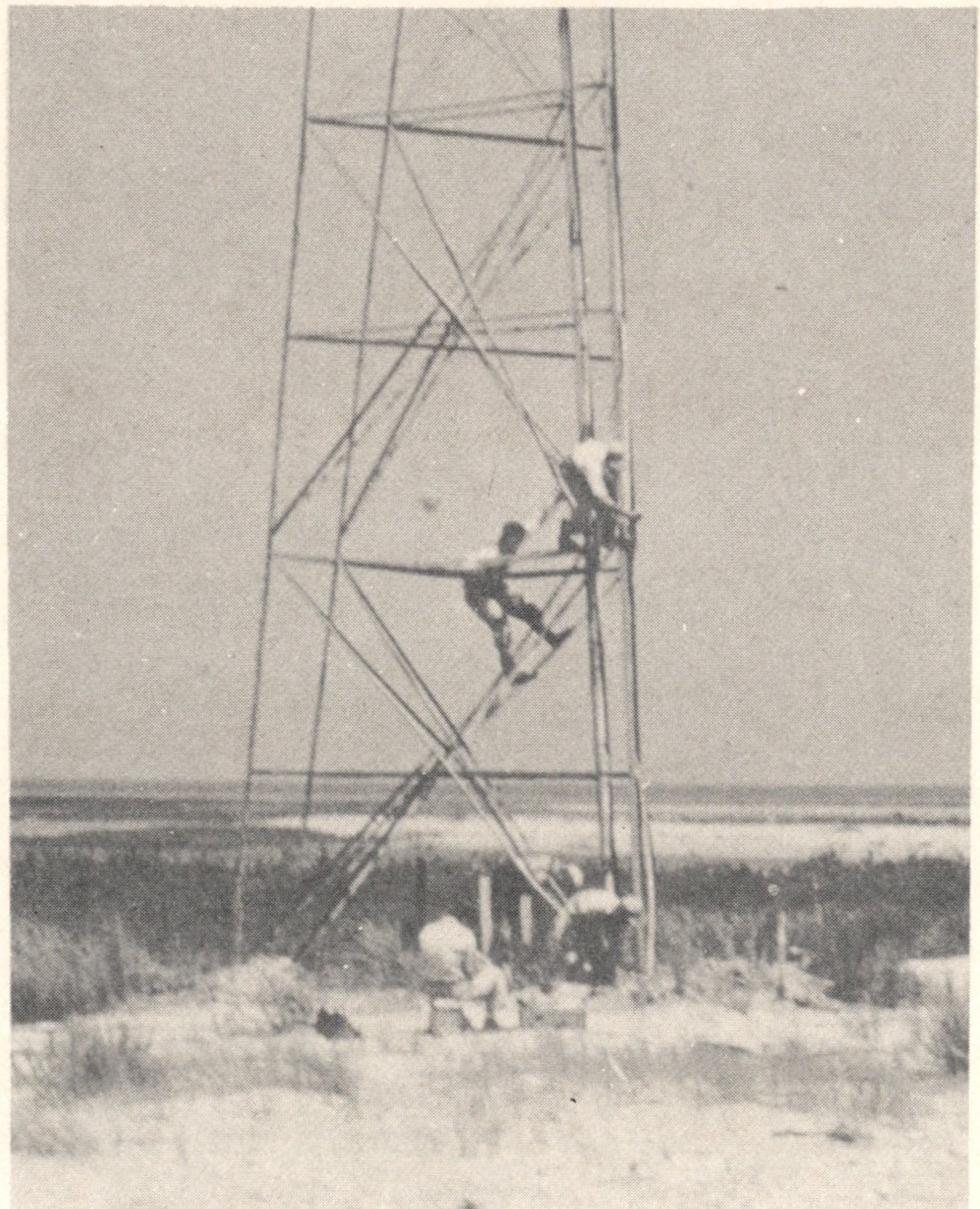
On shell banks such as this, the tower footings could be dug down about 1 foot.
