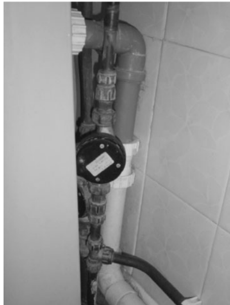
Plate 1 Telemetry meter fitted to bathroom sink
