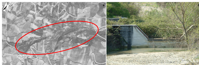
Fig. 6 Location of the remedial work visible on the historical aerial reconstruction (a); details of the concrete weirs built along the tributary of the Verrino Creek (b)
