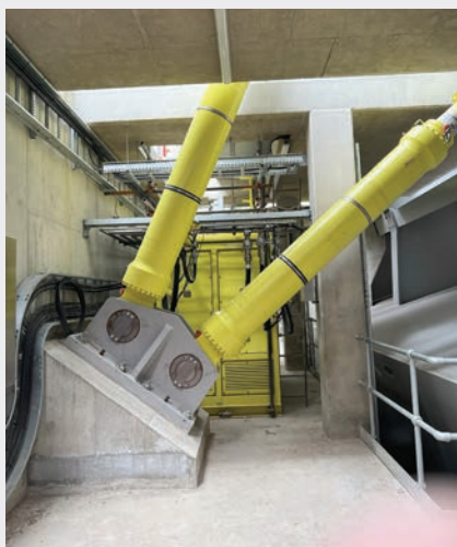
LIEBIG Ultraplus anchors securely angled to support the hydraulic mechanisms of the bridge decks as well as the tail locks that hold the Herring Bridge in its raised and open position.
