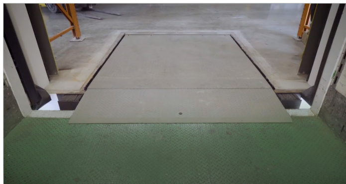
A pit-style leveler creates a smooth transition from the dock floor to the trailer bed
