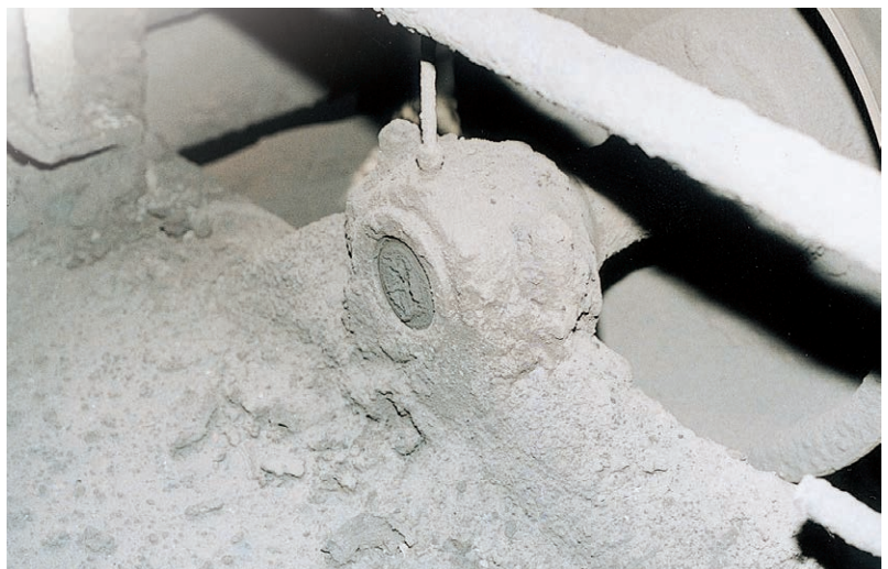
Pulley bearing in extreme contamination conditions (Plummer block)
