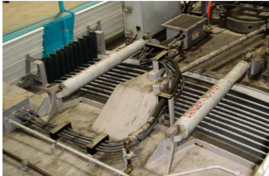
FIGURE 6 Roof-mounted dampers and Z-links, Santa Clara VTA cars.
