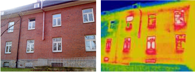
Fig. 8.15: Photo of eight windows (left) and the corresponding infrared image (right). In the thermal image heat losses are clearly detectable. In the top row the windows show different temperature distributions. The first window on the left belongs to an empty office which is not heated. The top part of the second window is open. The third window is closed and has proper insulation. The fourth window shows unusually high temperatures. This was caused by a partially detached rubber insulation strip that allowed the air to flow through.
