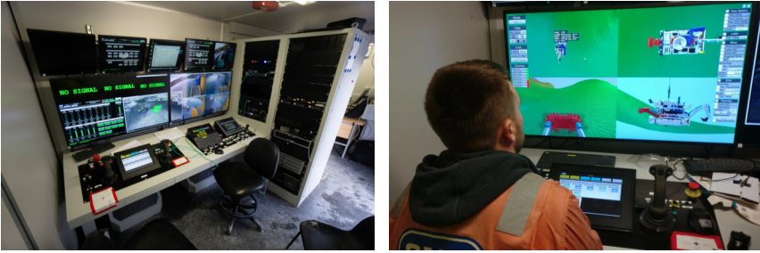
Fig. 7.6: The control cabin has two work places: one for the operator of the mining vehicle and one for the operator of the LARV and slurry circuit.
