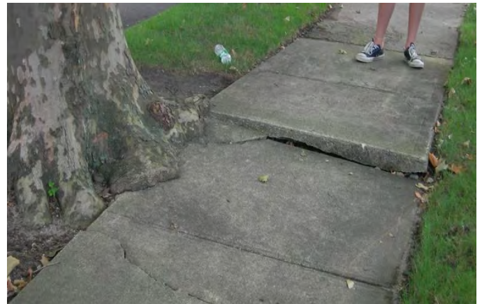
The roots of this tree have grown through the compacted soil beneath the sidewalk, into the large volume of soil beyond. Expanding tree roots have caused the sidewalk to heave.
