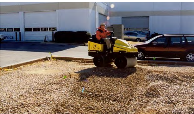
Compaction of CU-Structural Soil® prior to installing sod. Photo courtesy Southpine, Inc.
