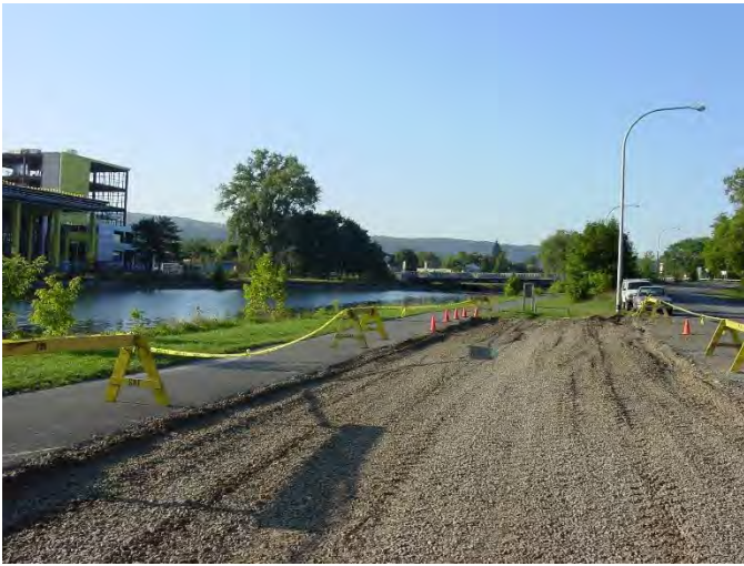
CU Structural Soil® was used as a 2' deep base course for the entire parking lot
