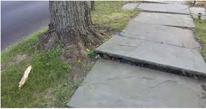
Tree roots heaving pavement
