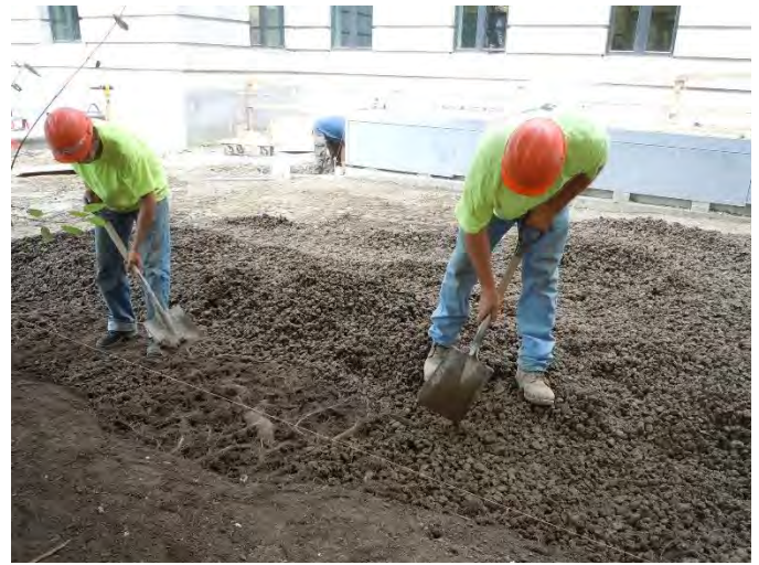
12"-15" of CU-Soil® was placed on top of the exposed roots and compacted for use as a base course for the paving
