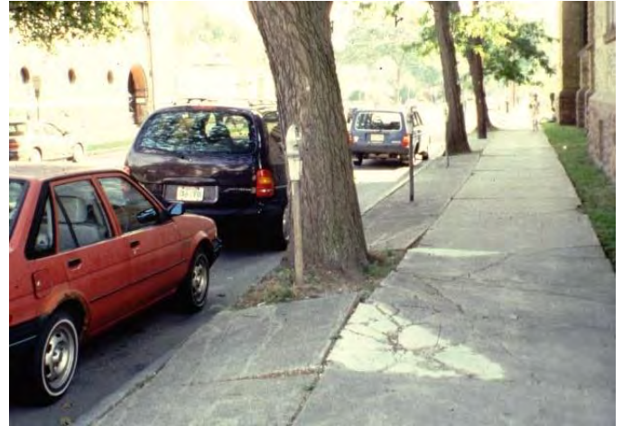
Trees planted in severely limited soil volumes die young unless their roots are able to break past compacted soils into an adequate volume of useable soil. This often results in dangerous sidewalk heaving.
