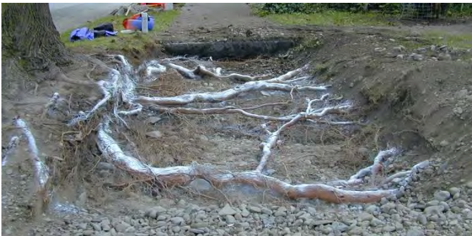
Thick superficial roots that have caused a sidewalk to heave.
