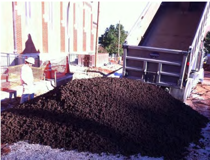
CU-Structural Soil® being delivered to project site. Photo courtesy Minick Materials Company
