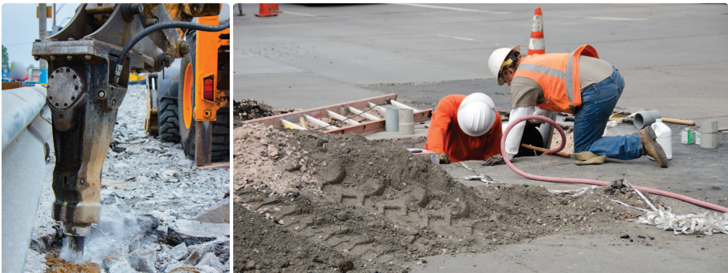
Left: Excavation equipment breaks up concrete as part of road repair project. Right: Workers pull electric cables underground during construction project in Denver, Colo.
