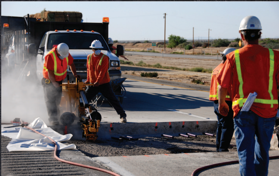
Highway construction crews work to replace a section of the roadway as part of ongoing road maintenance projects.
