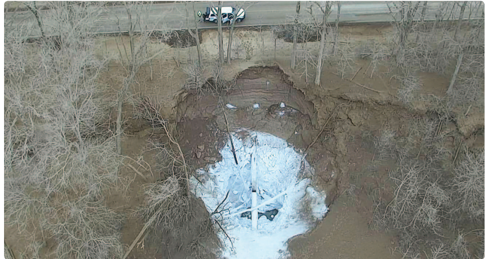
Carbon dioxide pipeline rupture in Satartia, Mississippi. Photo credit: Mississippi Emergency Management Agency.
