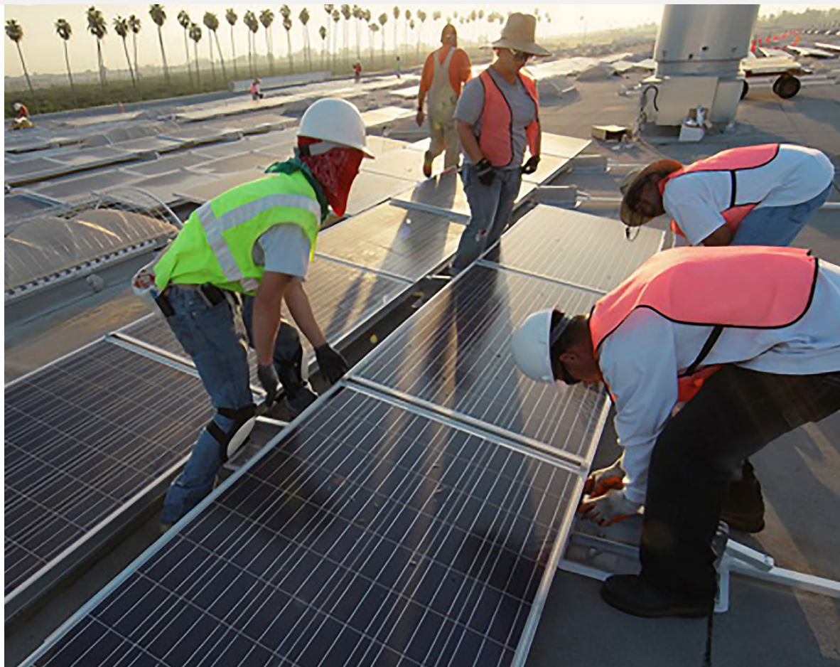
Solar panels at a Prologis property in Redlands, California.
