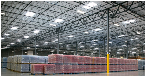
LED installation at LEED Gold-certified Prologis Park Cheyenne, Las Vegas, Nevada.
