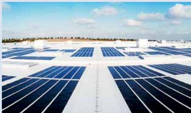
Solar Panels at ProLogis Park Chanteloup (Moissy-Cramayel, France)
