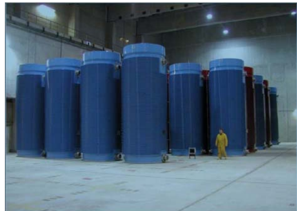
Figure 3: Storage hall with storage casks
