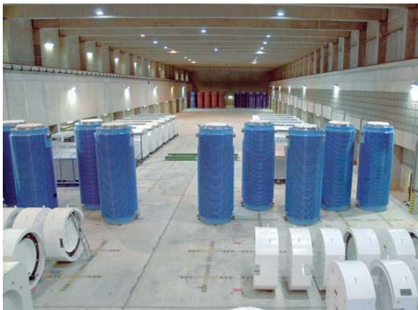
Figure 2: Storage hall with newly arrived casks and shock absorbers in the foreground
