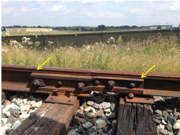
Figure 2. Photograph of an exemplar compromise joint bar denoted by arrows (not Metro-North).
