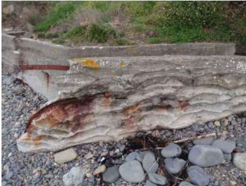
Western side of position shows sandbag construction method prior to pouring concrete, also note steel reinforcing
