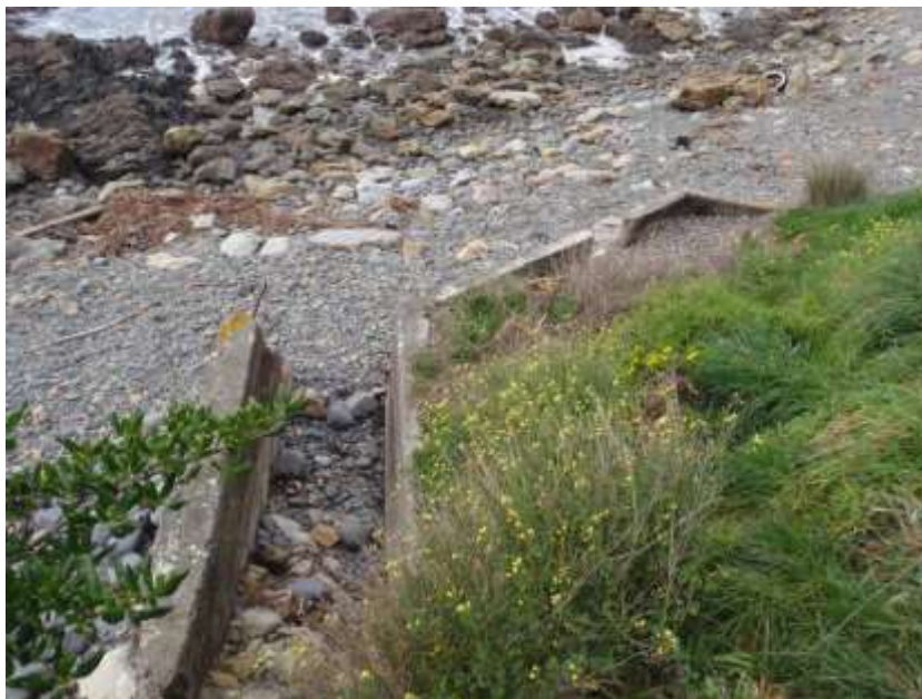
Intact portion of 'trench' on western side as viewed from walking track above.
