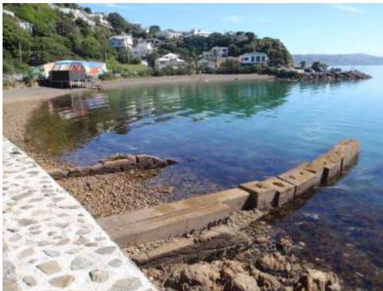
Figure 96: Concrete groins constructed for beach protection at southern end of Balaena Bay
