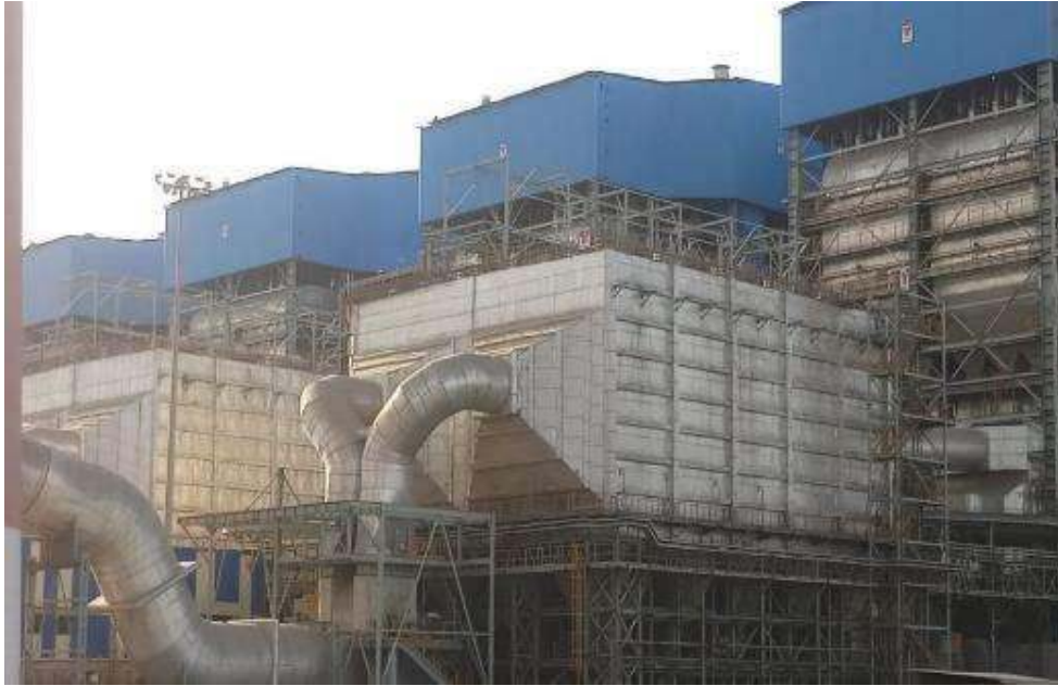
ESP's Installed at CCPP
