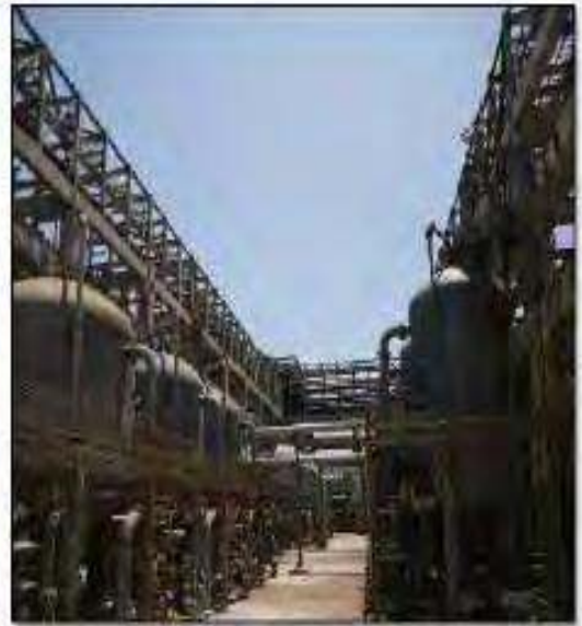
MEDIA FILTRATION SYSTEM
