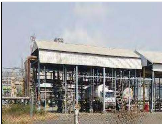
Loading Arms at Tank Farm
