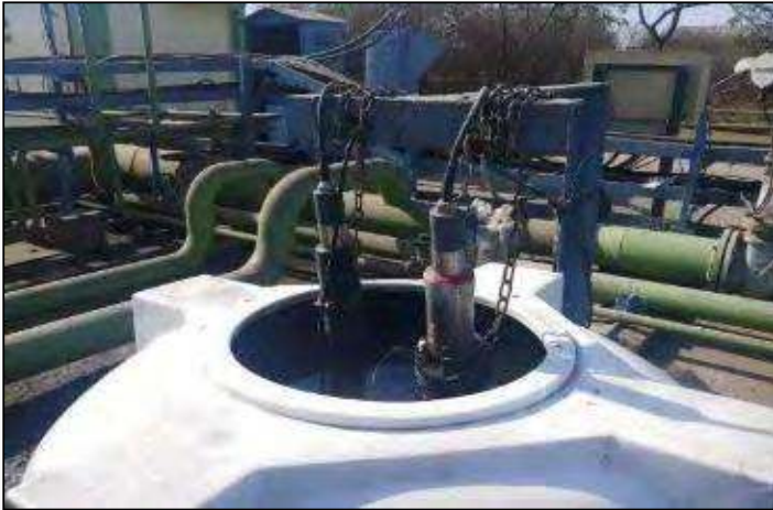
Analysers of Continuous Effluent Monitoring System installed at outlet
