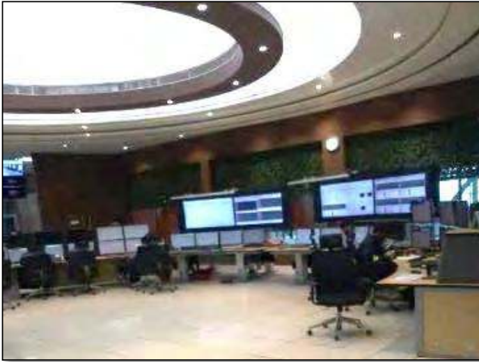
Photograph of State of the art Control Room equipped with DCS
