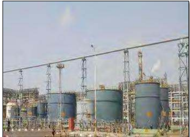
MEG / DEG Storage Tanks
