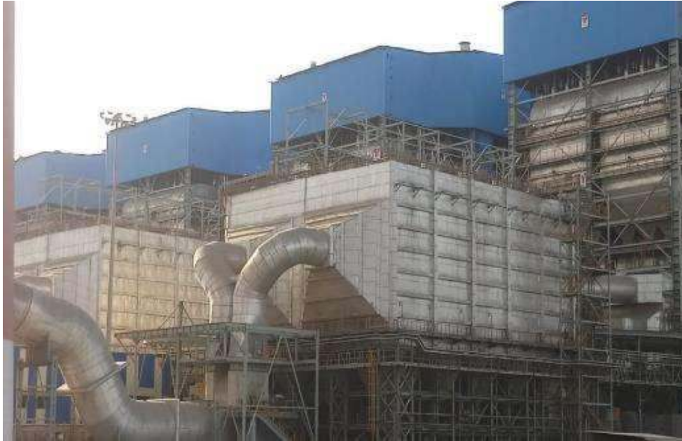
ESP's Installed at CCPP
