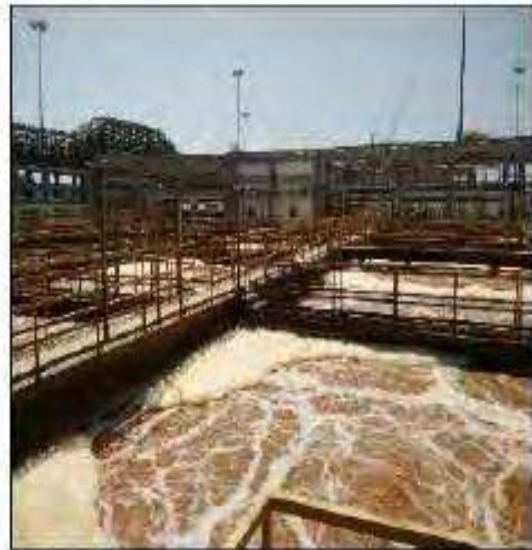
MBR Aeration Tank
