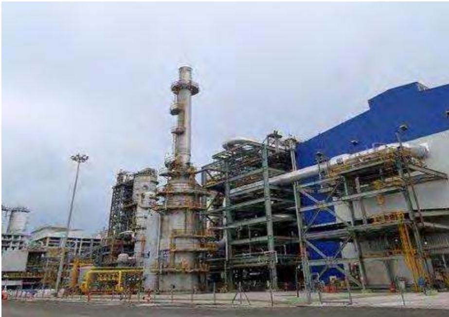
Stack attached with Off Gas Scrubber in PTA Plant
