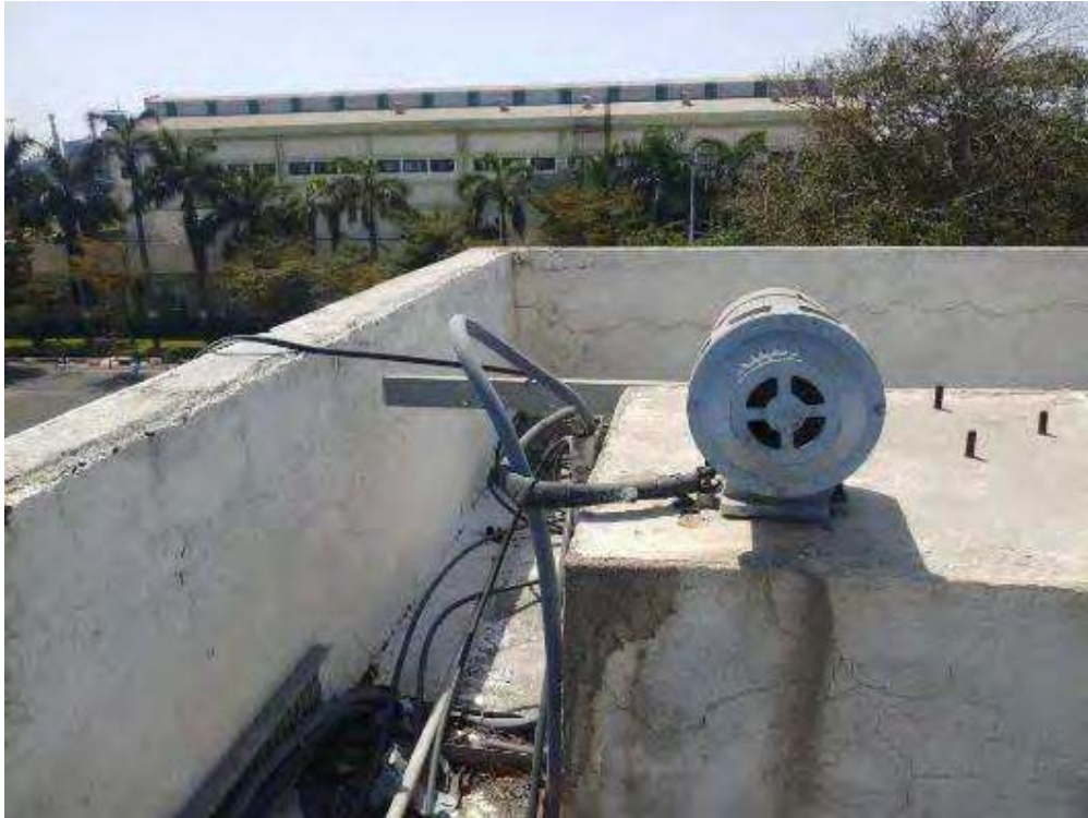
Photograph of Siren installed at SSM Building
