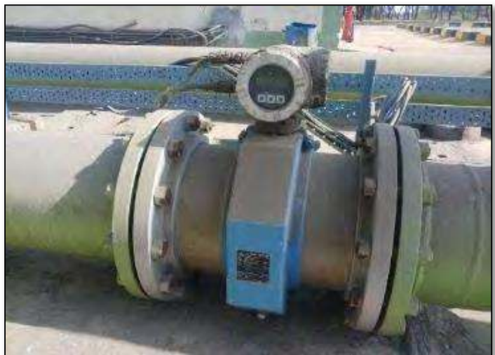
Flow Meters installed at ETP outlet
