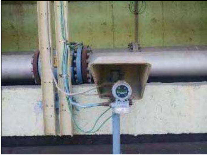
Flow Meters installed at ETP inlet
