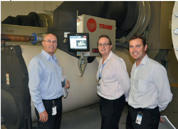
(L-R) Gold Coast Health Maintenance Coordinator Barry Walker with Nigel Hoy and Siemens Building Engineering and Maintenance Manager Shane Berryman. Image: Siemens.
