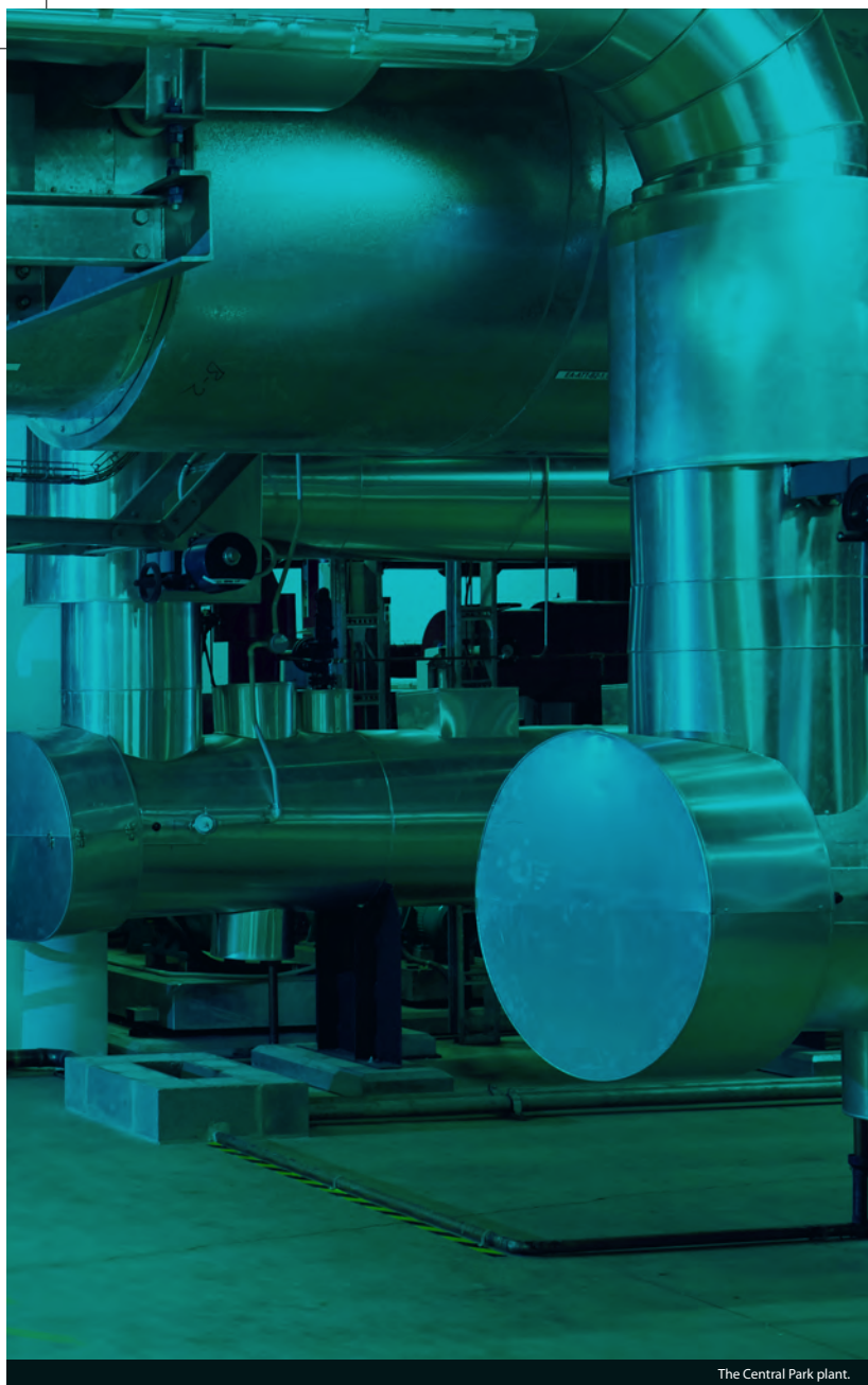
The Central Park plant.
