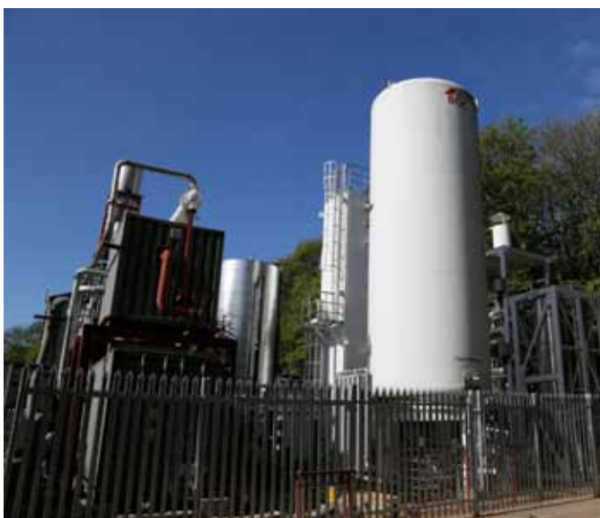
Experimental cryogenic energy storage facilities at the University of Birmingham.
